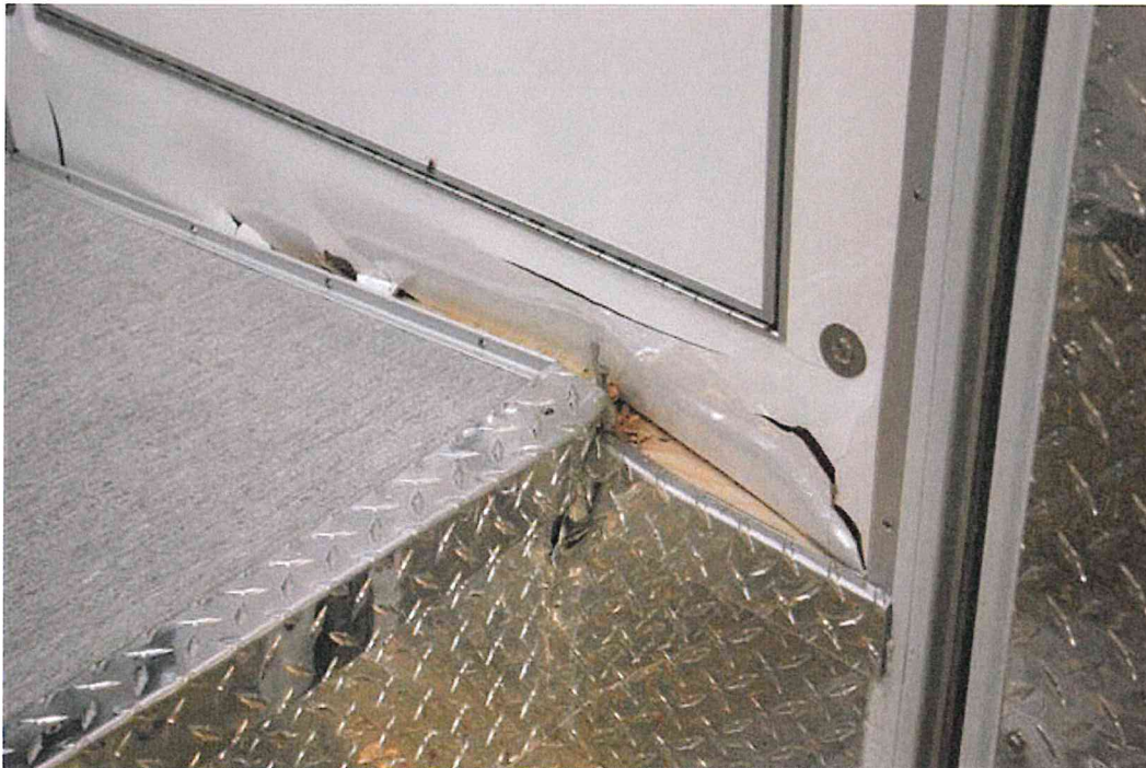
VIEW SHOWING DAMAGE INSIDE PERSONNEL DOOR (TEST 052)
