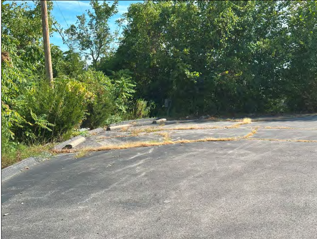
Osage Village Inn – deterioration of pavement; overgrown vegetation (TIF Study Area only)
