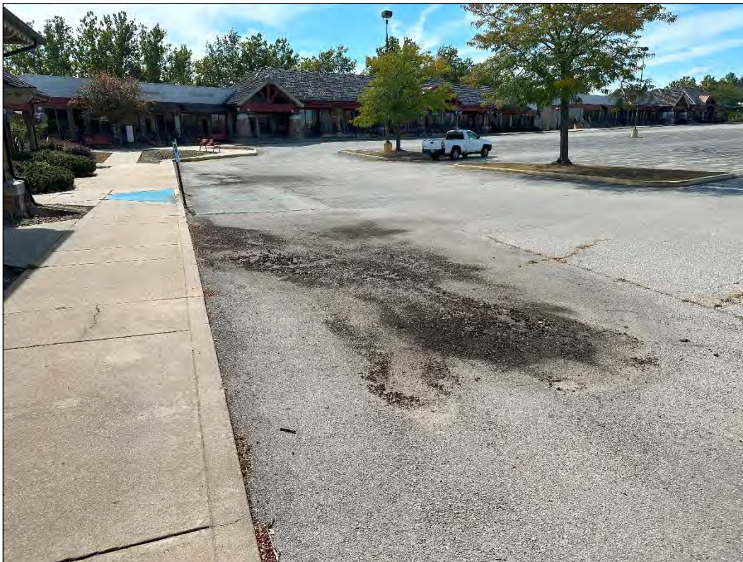
4540 Osage Beach Pkwy – deterioration of pavement
