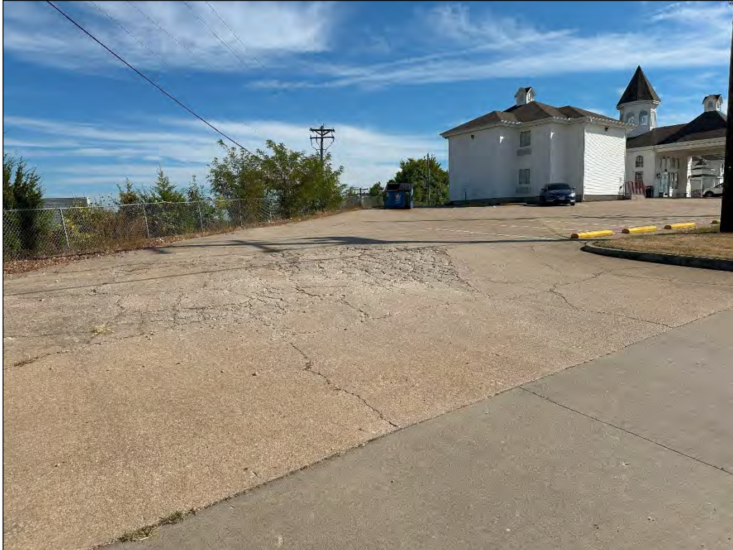
Osage Village Inn – deterioration of pavement (TIF Study Area only)
