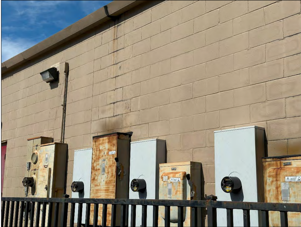
4540 Osage Beach Parkway – deterioration of equipment, gutter; failure of finishes
