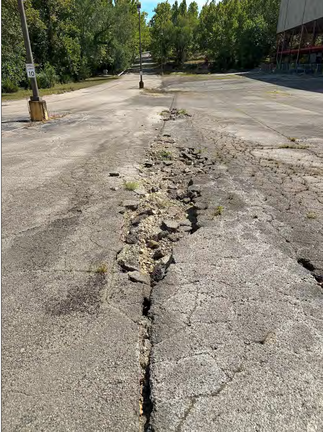
4540 Osage Beach Pkwy – deterioration of pavement
