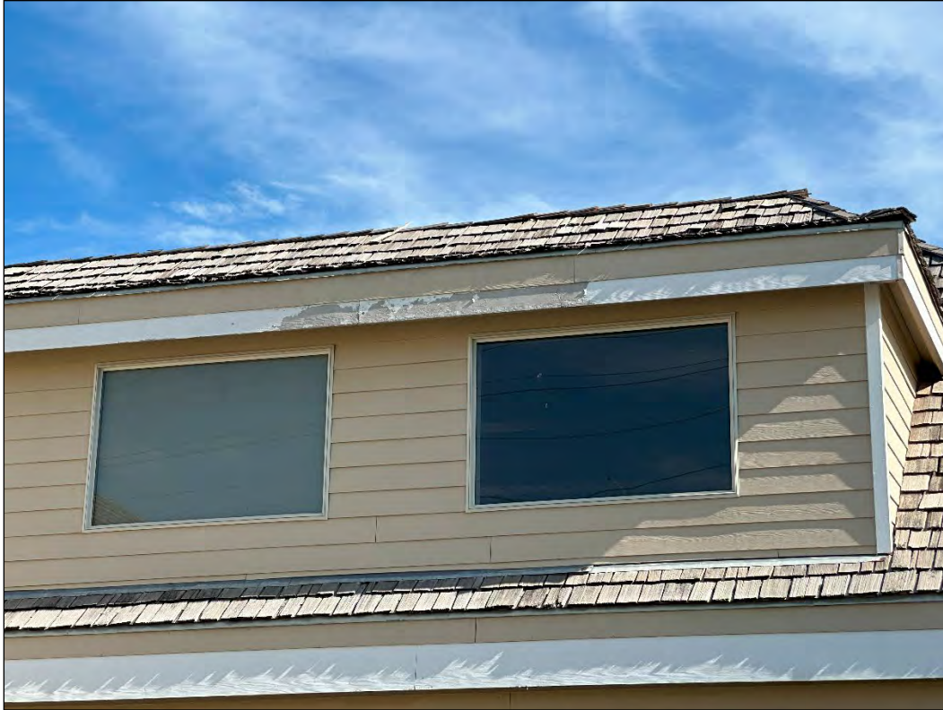
First Bank Office Centre – deterioration of finishes, shake shingle roof (TIF Study Area only)
