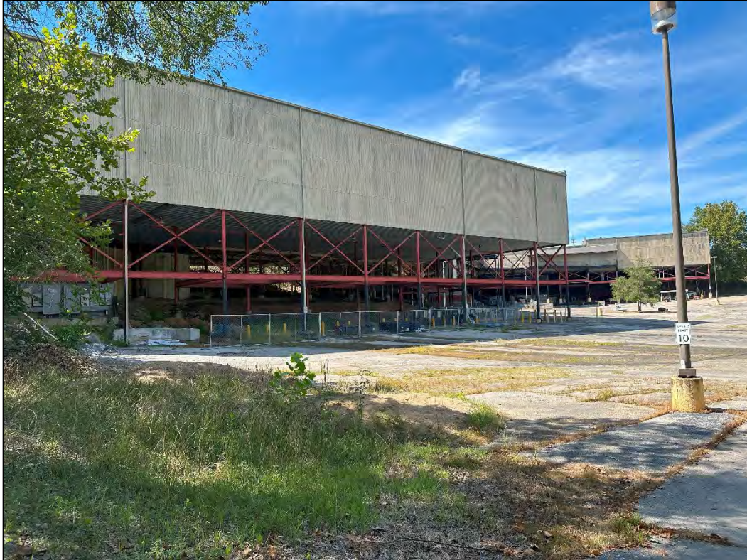
4540 Osage Beach Parkway – fencing erected to prevent access to corroded steel walkways and stairs
