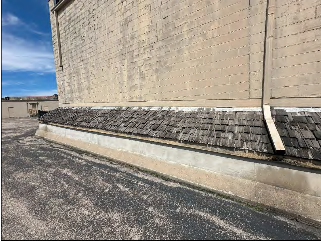
4540 Osage Beach Parkway – failure of finishes; deterioration of wood shake shingles, downspouts
