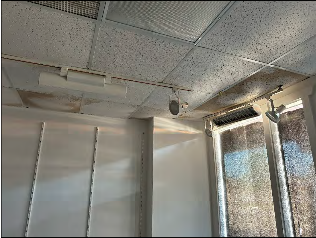
4540 Osage Beach Parkway – evidence of water damage caused by leaking roof/burst pipe
