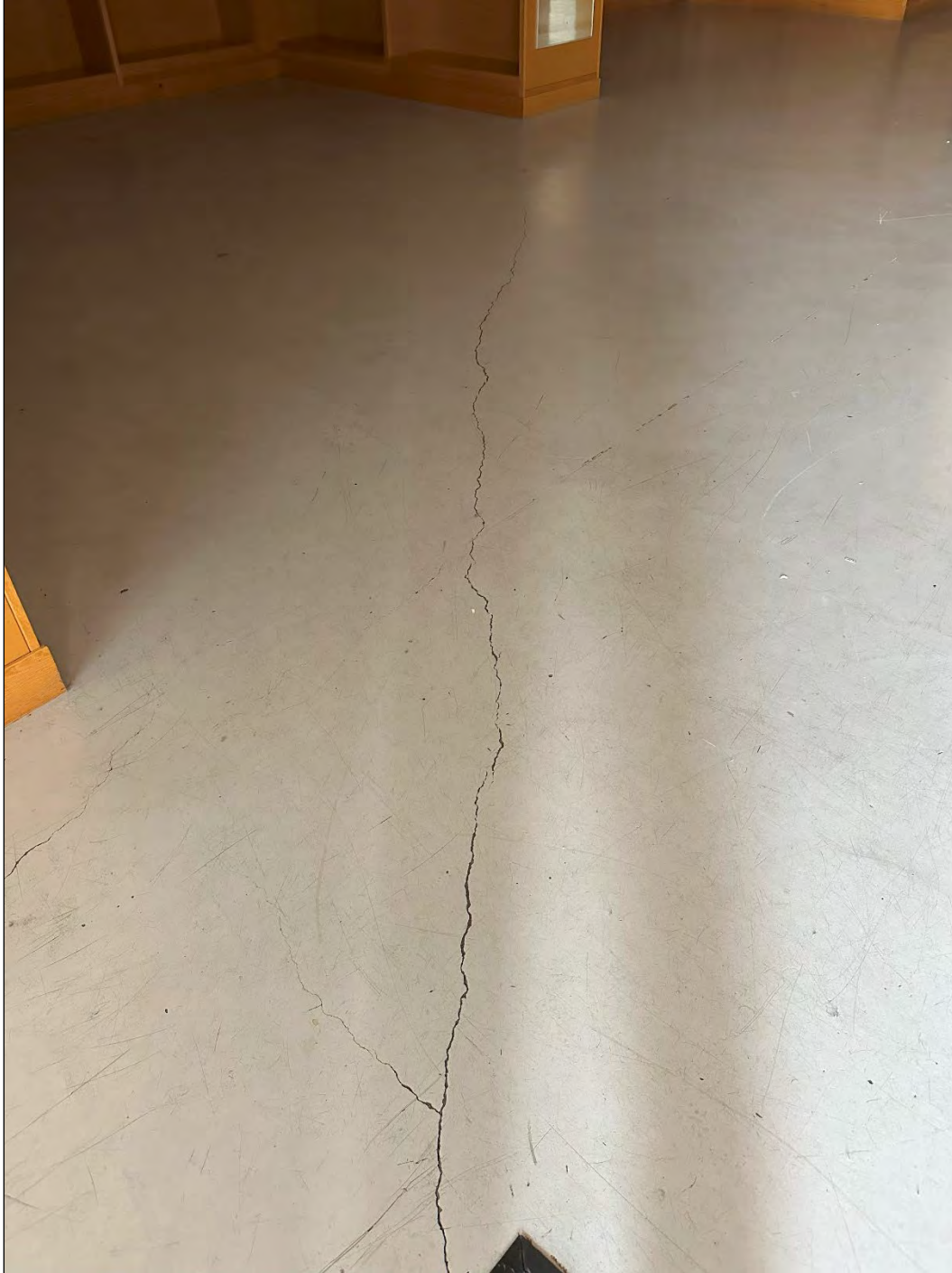
4540 Osage Beach Parkway – structural cracking in floating slab (interior of retail space)
