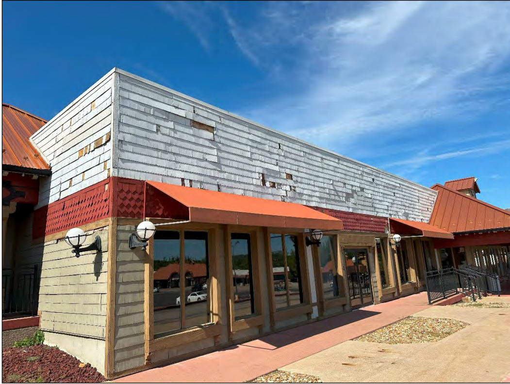
4540 Osage Beach Parkway – deterioration of wood siding; failure of finishes, light fixtures
