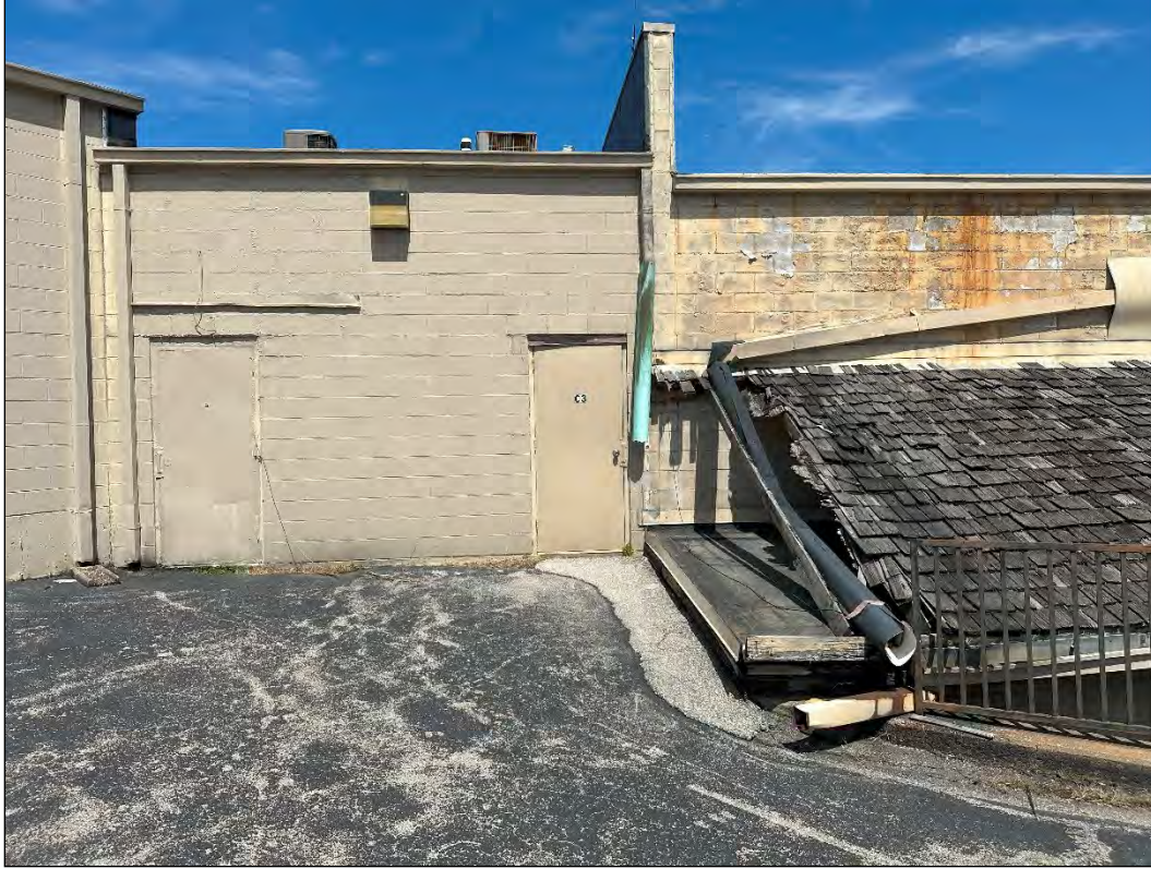
4540 Osage Beach Pkwy – deterioration of shake shingle roof, downspouts; failure of finishes
