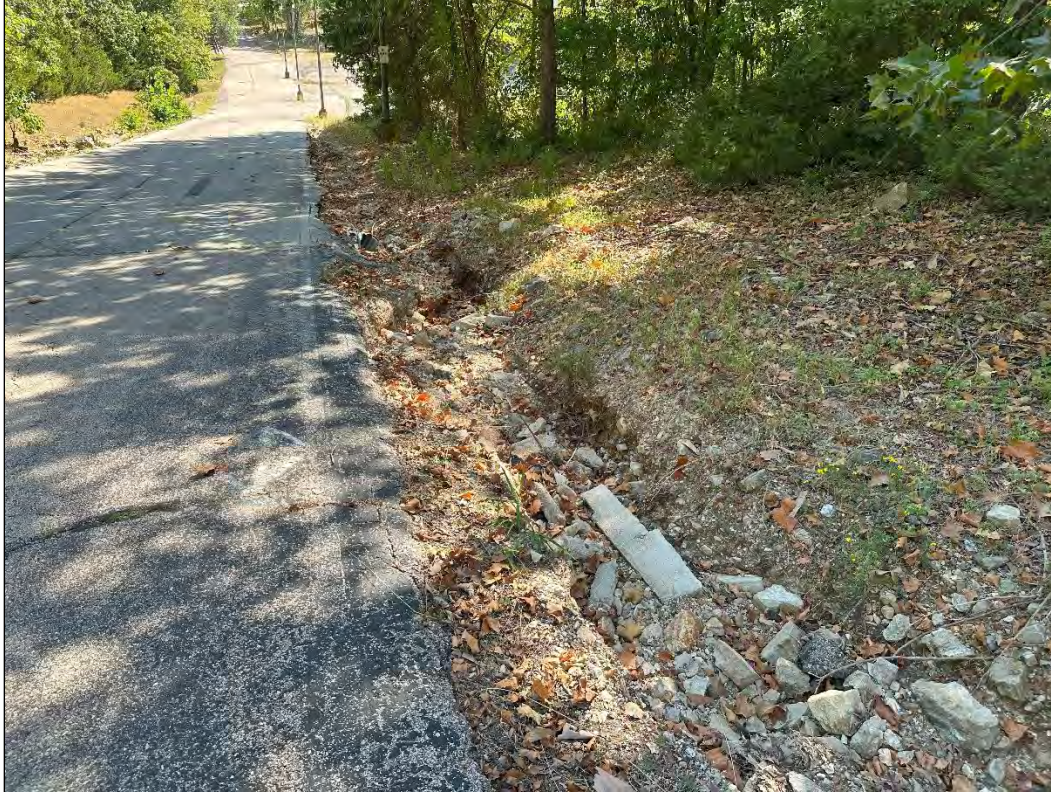
4540 Osage Beach Parkway – poor drainage, deterioration of service drive
