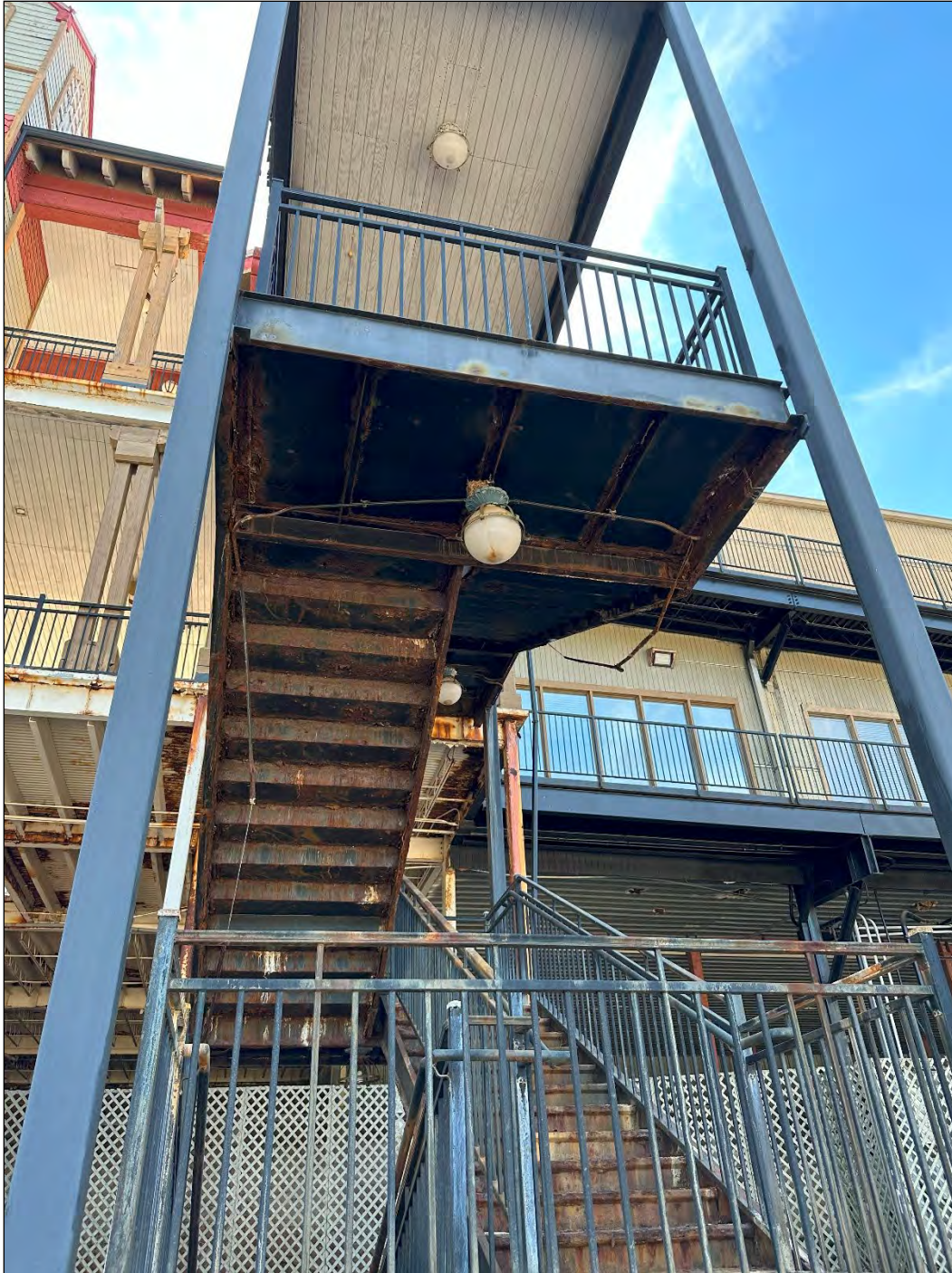
4540 Osage Beach Parkway – deterioration of stairs; failure of finishes
