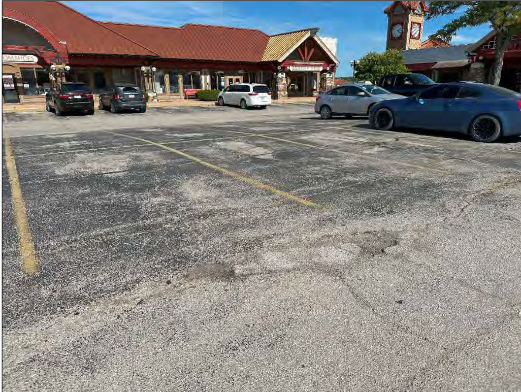
4540 Osage Beach Pkwy – deterioration of pavement
