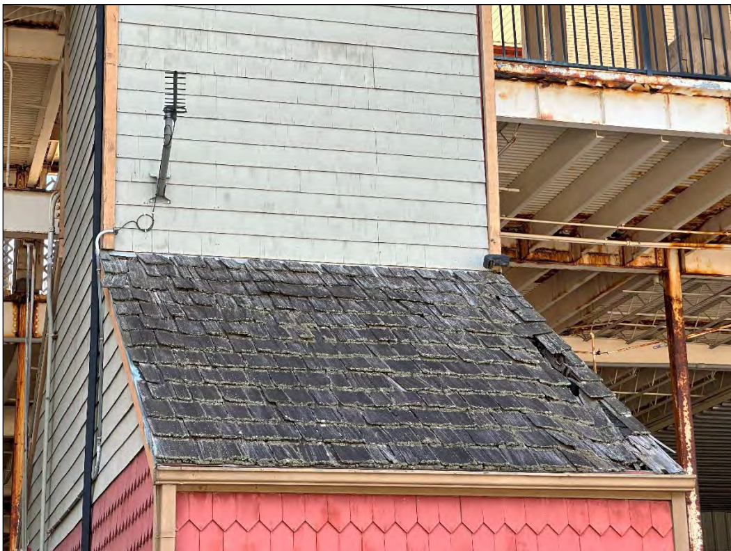
4540 Osage Beach Parkway – deterioration of shake shingle roof, siding; failure of finishes
