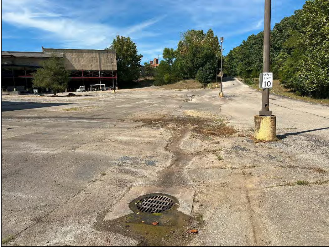
4540 Osage Beach Pkwy – deterioration of pavement
