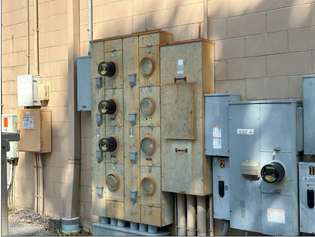
4540 Osage Beach Parkway – deterioration of equipment
