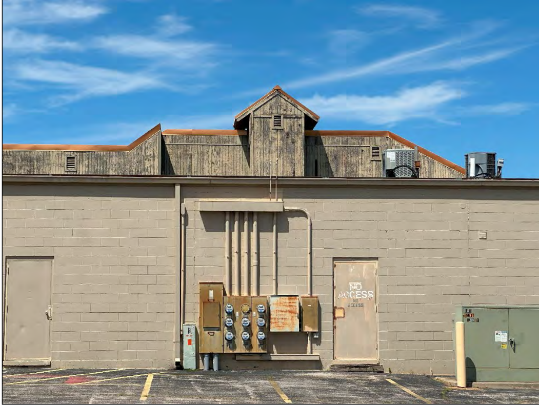
4540 Osage Beach Pkwy – deterioration of equipment, doors; failure of finishes
