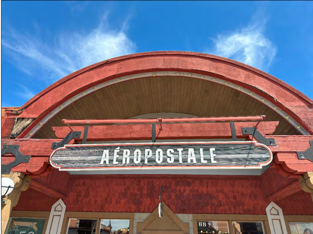
4540 Osage Beach Parkway – wood rot; failure of finishes
