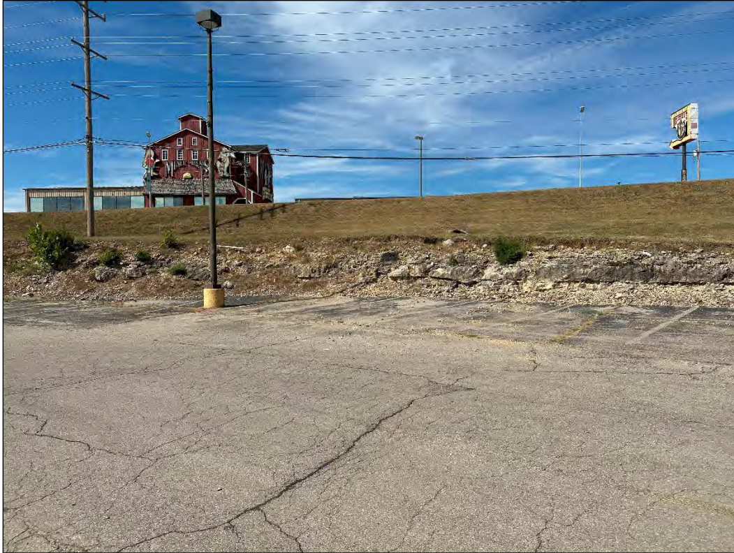
4540 Osage Beach Parkway – loose rock on parking surface
