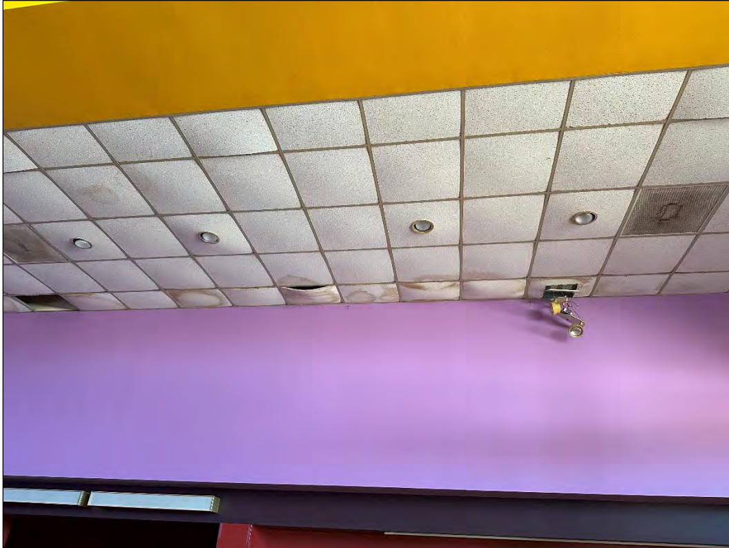
4540 Osage Beach Parkway – evidence of water damage caused by leaking roof/burst pipe
