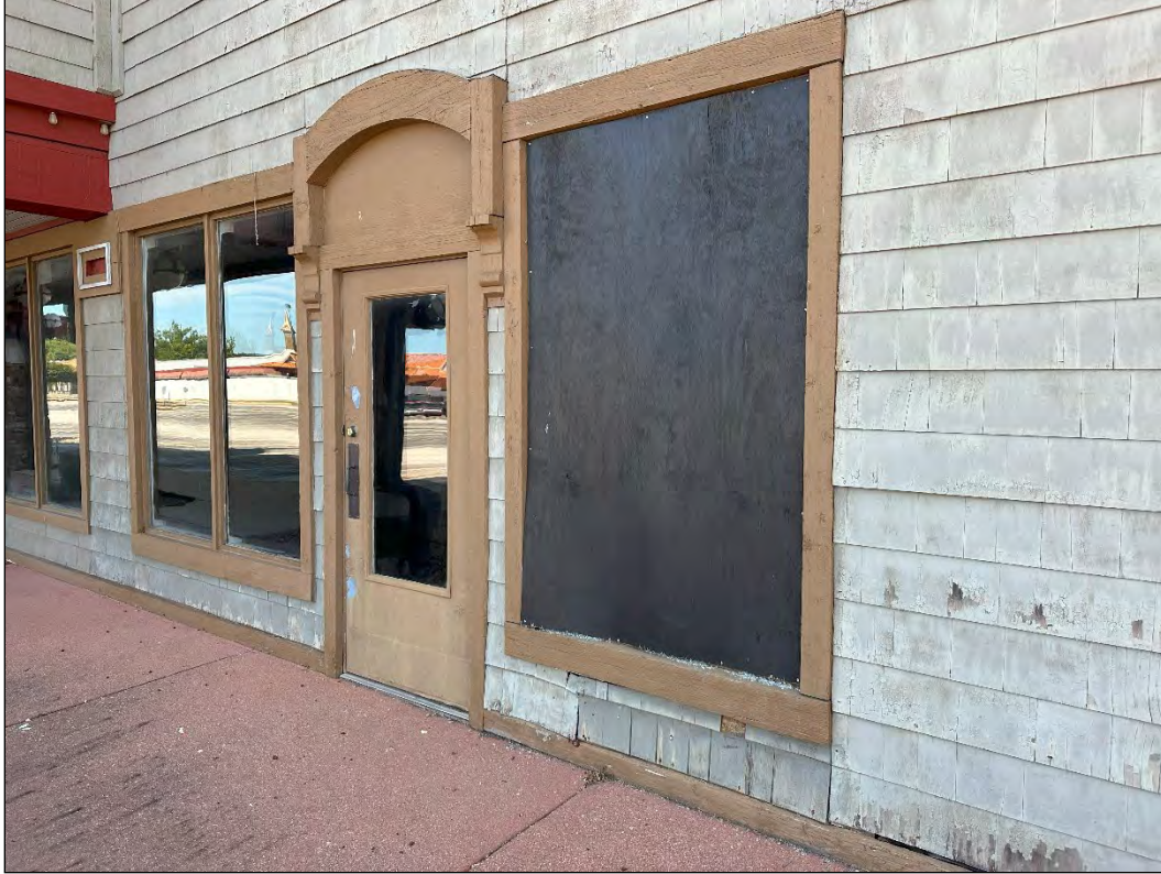
4540 Osage Beach Parkway – boarded broken window; deterioration of siding; failure of finishes
