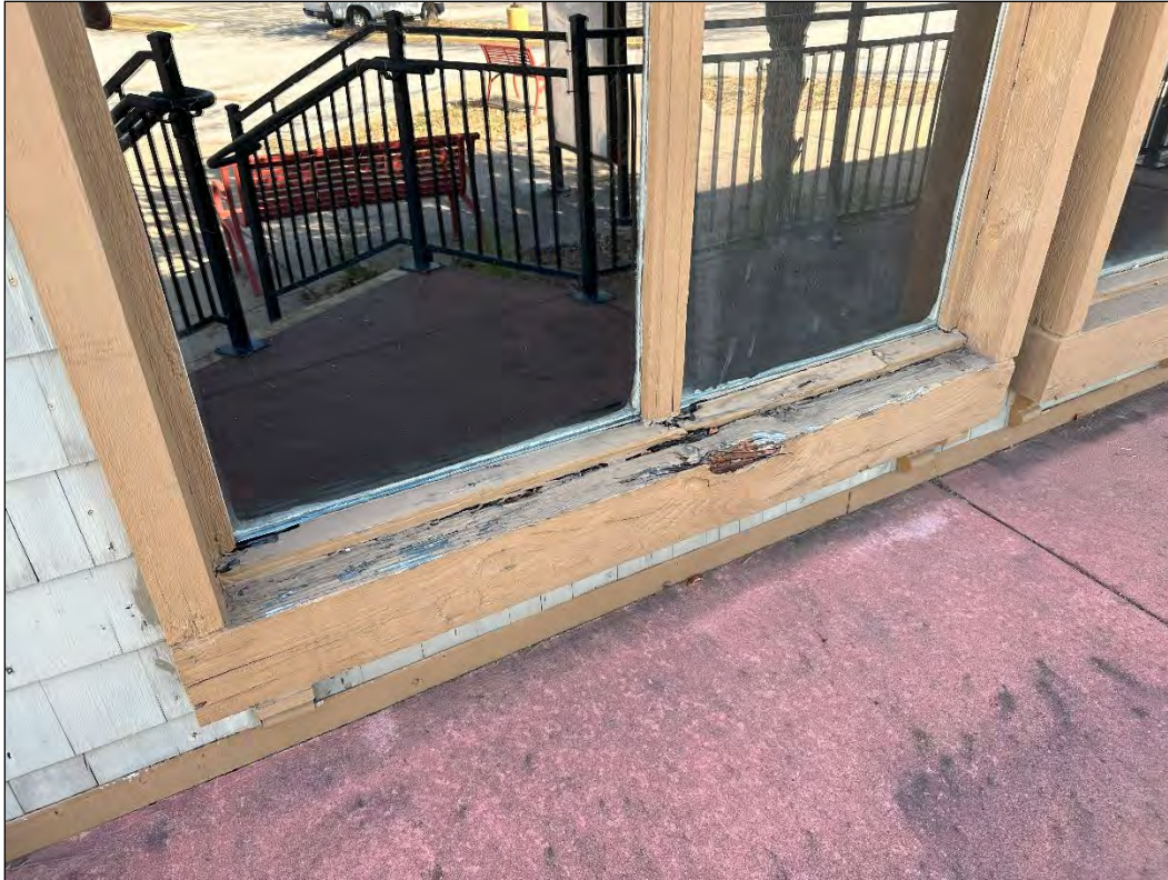
4540 Osage Beach Parkway – wood rot
