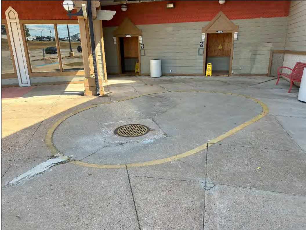
4540 Osage Beach Parkway – uneven pavement
