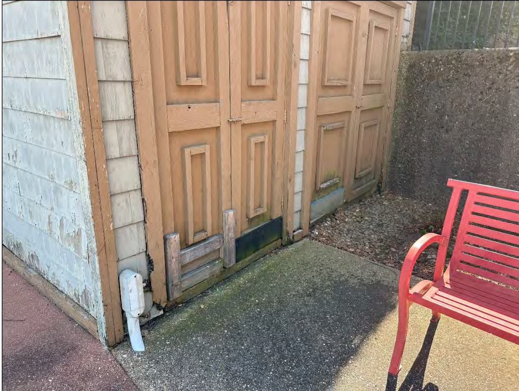
4540 Osage Beach Parkway – deterioration of doors, siding
