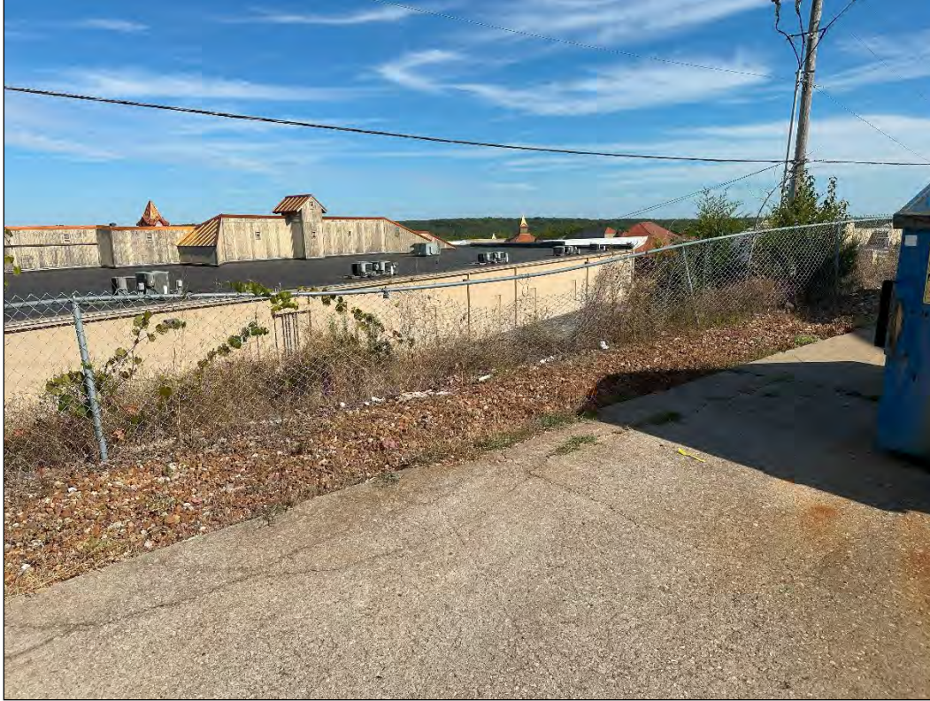
Osage Village Inn – deterioration of fence (TIF Study Area only)
