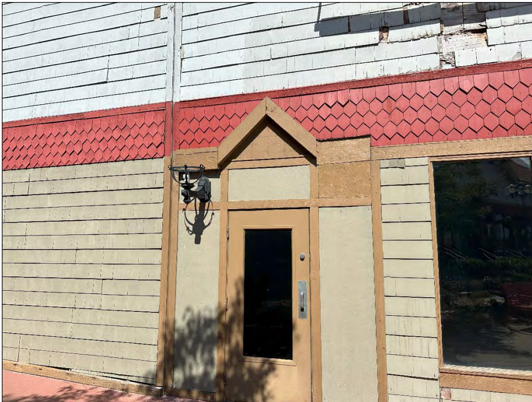
4540 Osage Beach Parkway – deterioration of siding; failure of finishes
