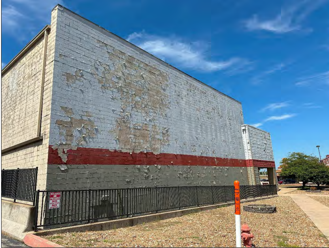
4540 Osage Beach Parkway – failure of finishes
