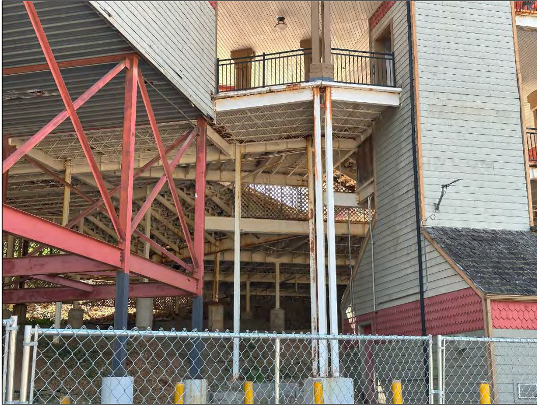
4540 Osage Beach Pkwy – deterioration of steel structure; failure of finishes
