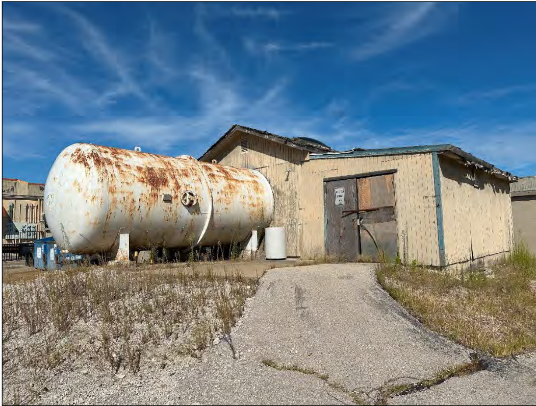
4540 Osage Beach Pkwy – deterioration of ancillary structure
