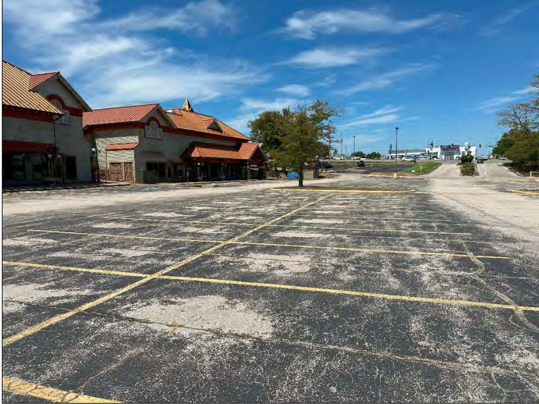
4540 Osage Beach Pkwy – deterioration of pavement
