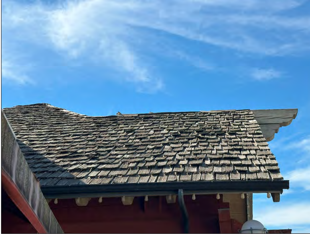
4540 Osage Beach Parkway – deterioration of shake shingle roof
