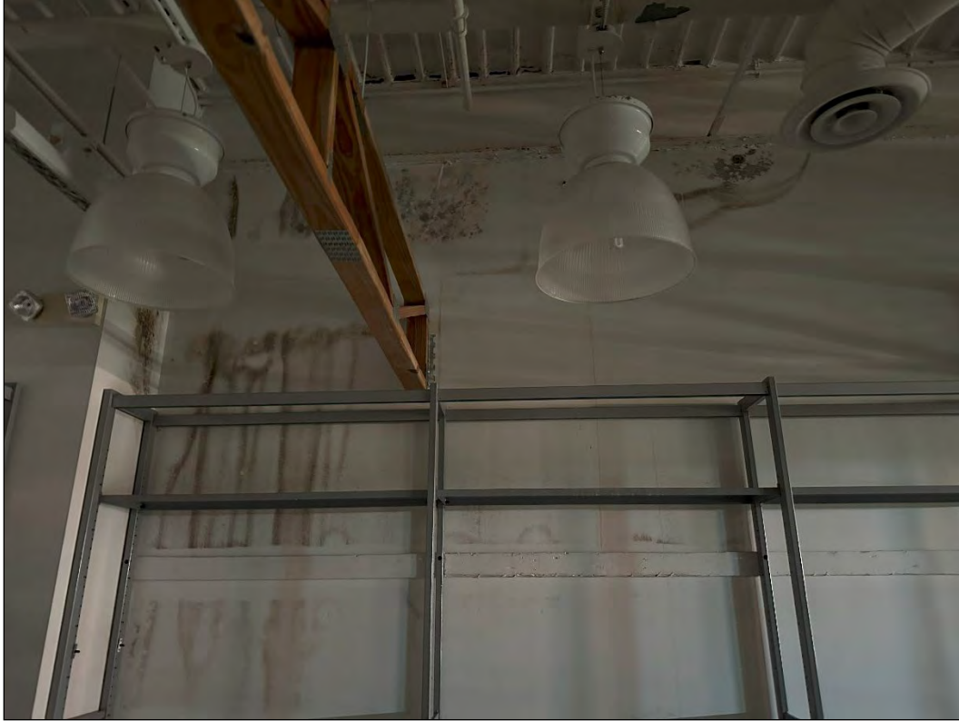
4540 Osage Beach Parkway – mold in retail space
