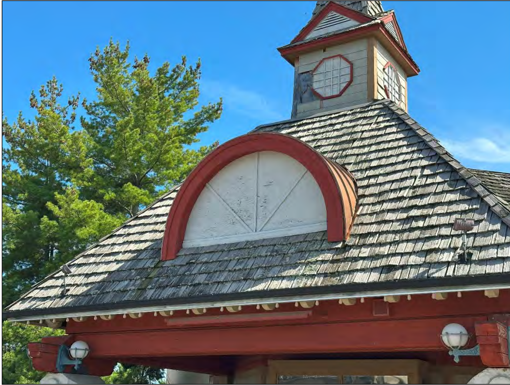
4540 Osage Beach Parkway – deterioration of shake shingle roof and siding; failure of finishes
