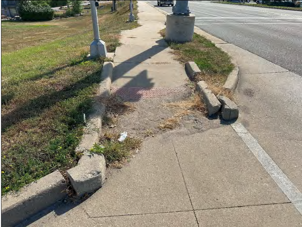
4540 Osage Beach Parkway – uneven pavement
