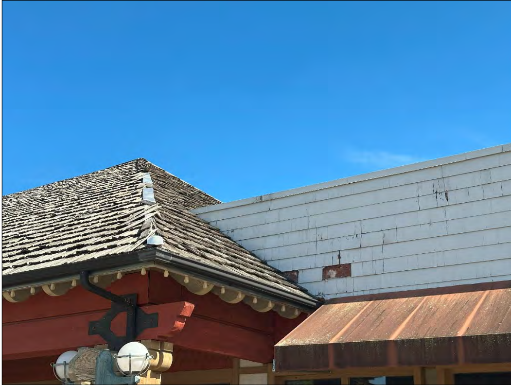
4540 Osage Beach Parkway – deterioration of shake shingle roof, siding, awning
