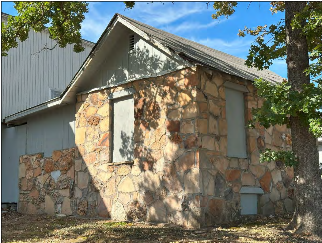
Quail's Nest – deterioration of ancillary structure
