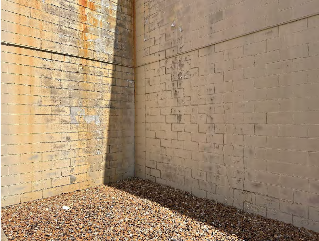
4540 Osage Beach Pkwy – deterioration of concrete block wall (cracking); failure of finishes
