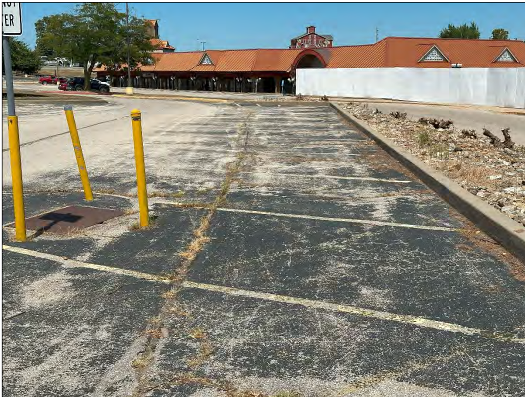
4540 Osage Beach Pkwy – deterioration of pavement; neglected landscaping
