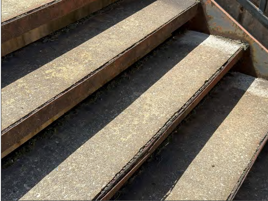
4540 Osage Beach Pkwy – deterioration of steps
