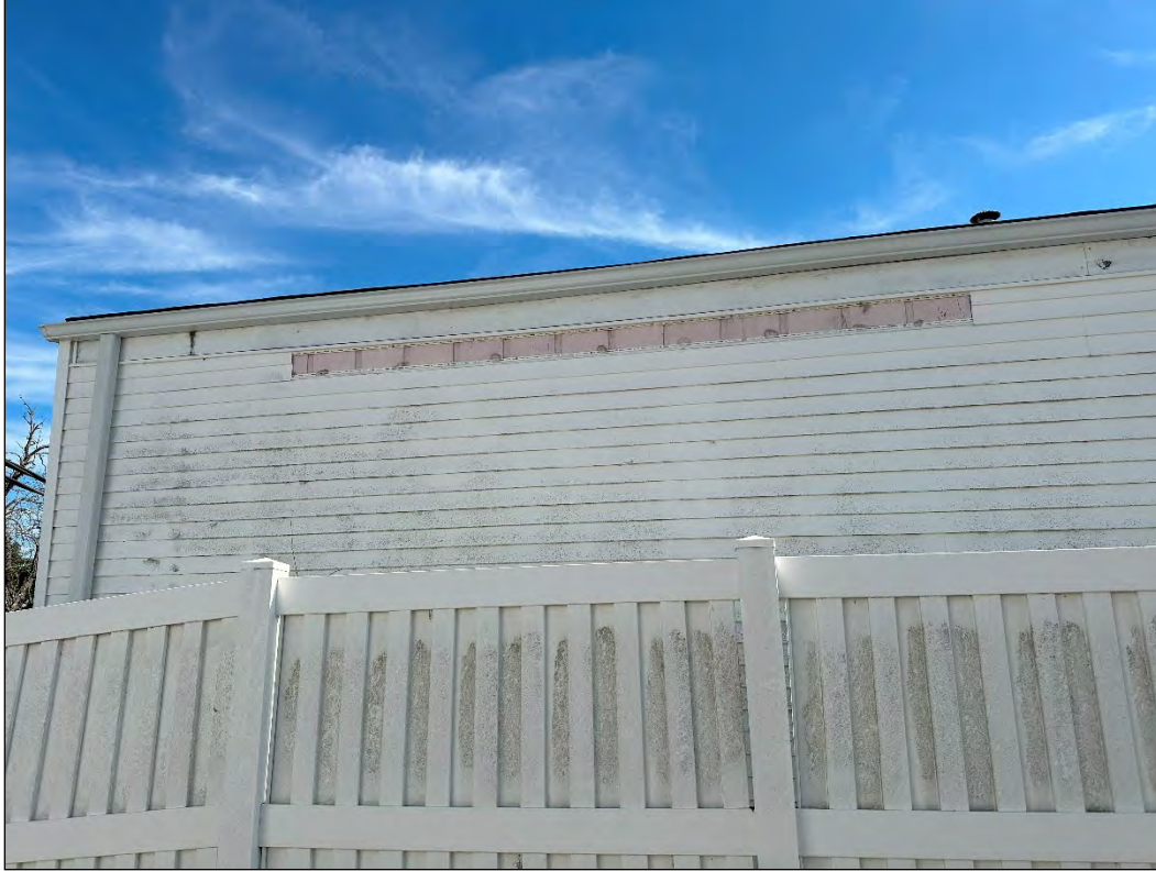
Quail's Nest – deterioration of siding, fence; failure of finishes
