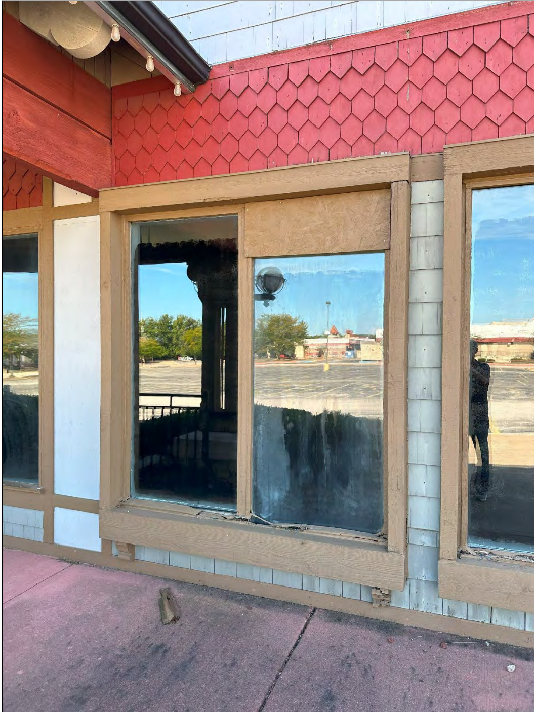
4540 Osage Beach Parkway – wood rot; broken window; deterioration of siding
