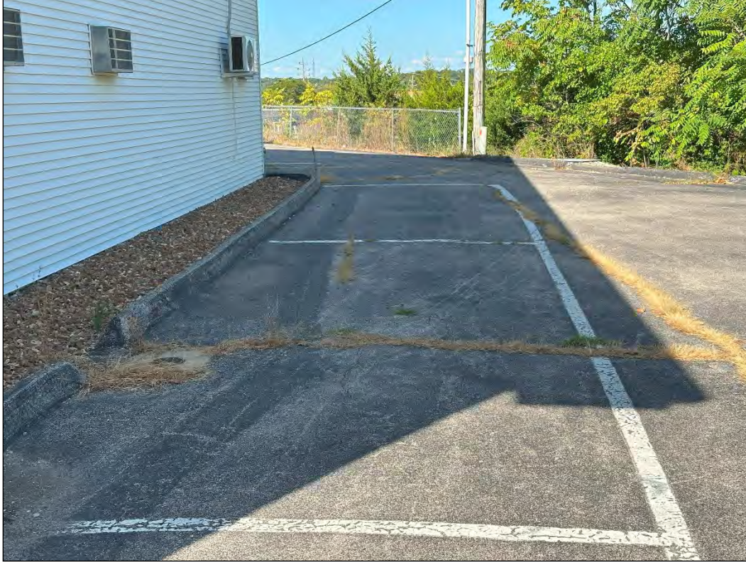
Osage Village Inn – deterioration of pavement; overgrown vegetation (TIF Study Area only)
