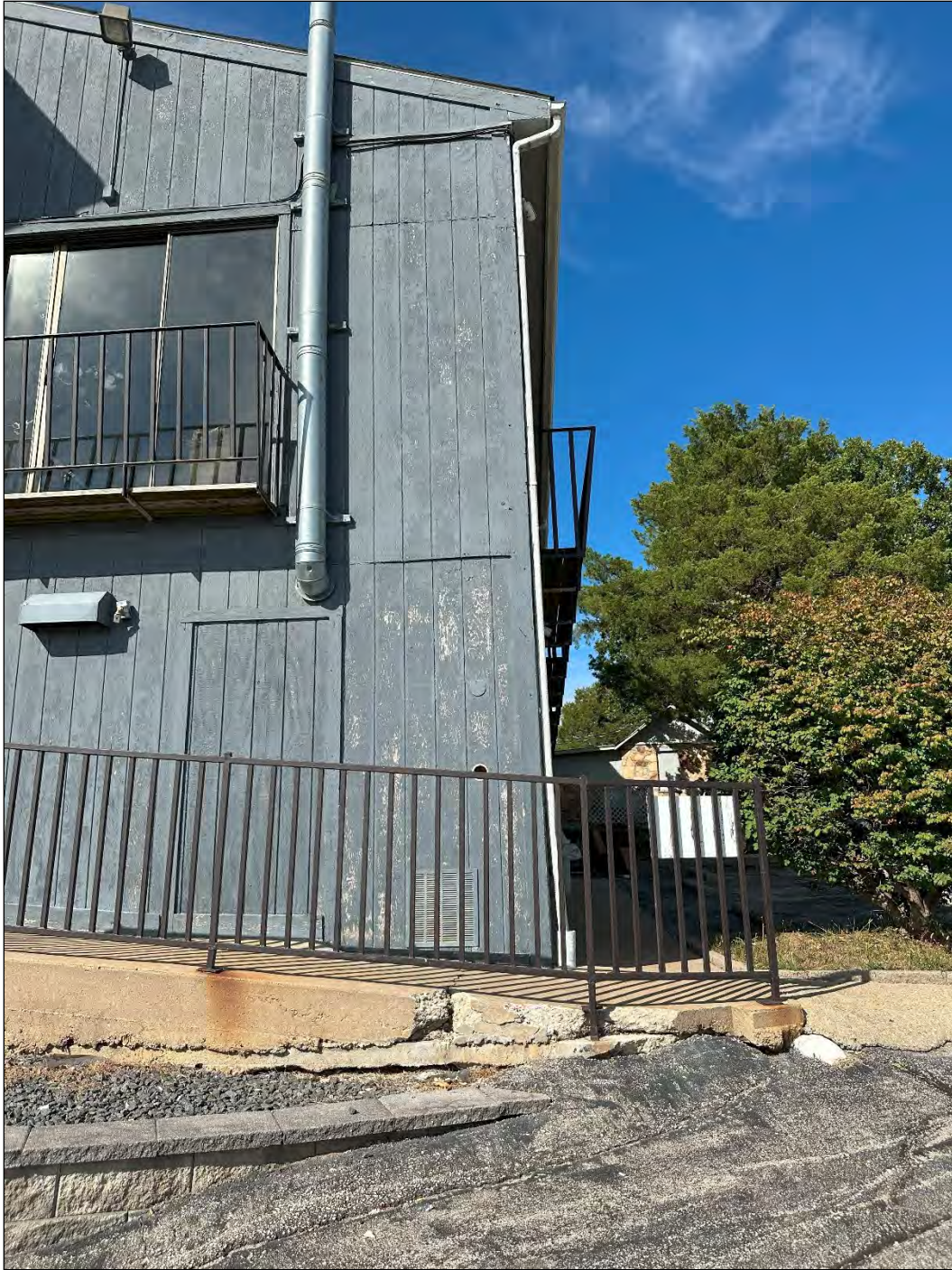
Quail's Nest – failure of finishes
