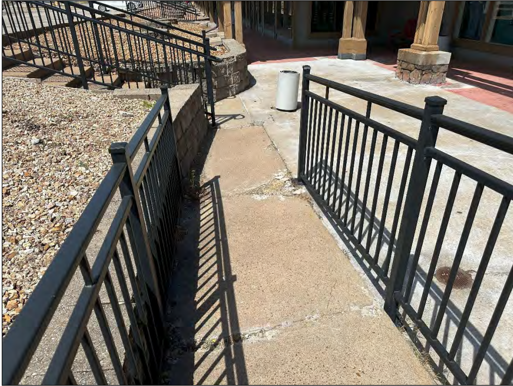
4540 Osage Beach Parkway – deterioration of walkway
