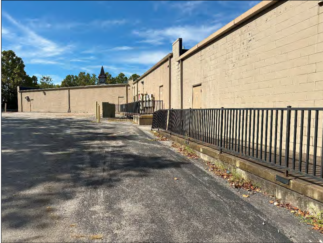
4540 Osage Beach Pkwy – deterioration of railing
