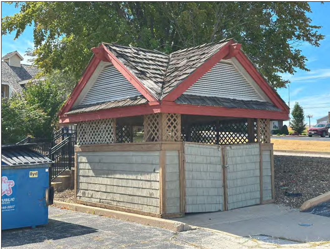
4540 Osage Beach Pkwy – deterioration of ancillary structure
