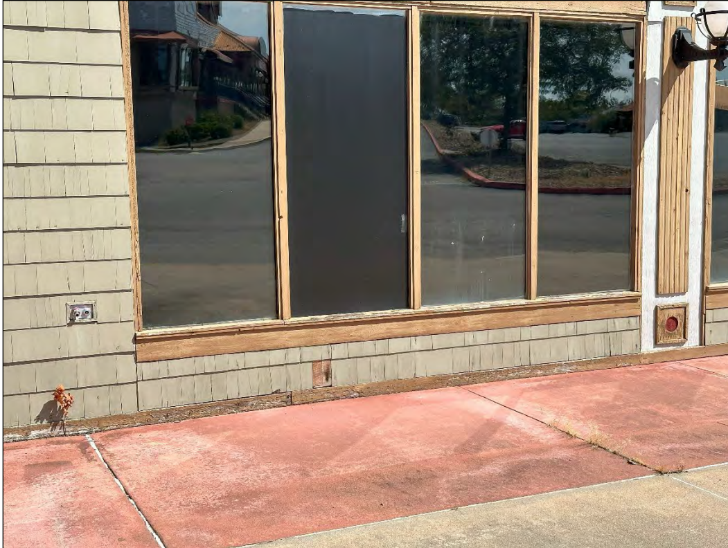
4540 Osage Beach Parkway – boarded broken window; wood rot; deterioration of siding, trim
