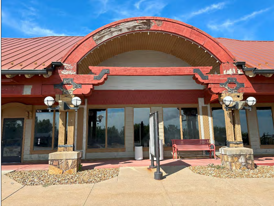
4540 Osage Beach Parkway – wood rot; failure of finishes; deterioration of light fixture supports
