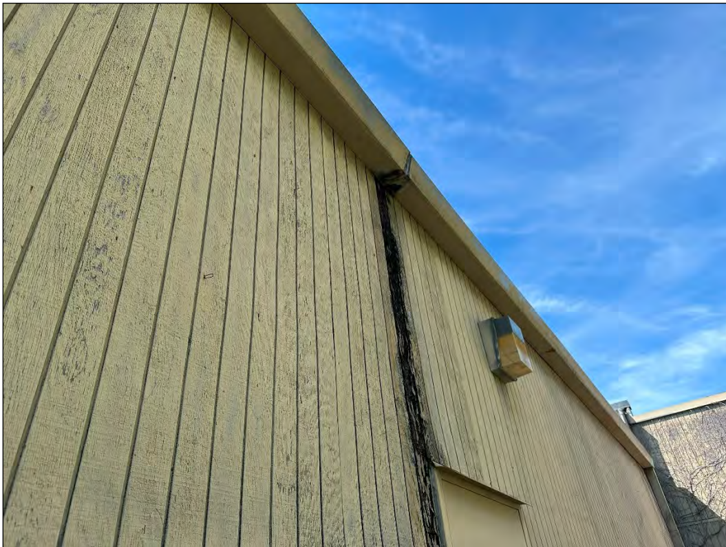
4540 Osage Beach Parkway – deterioration of gutter; failure of finishes
