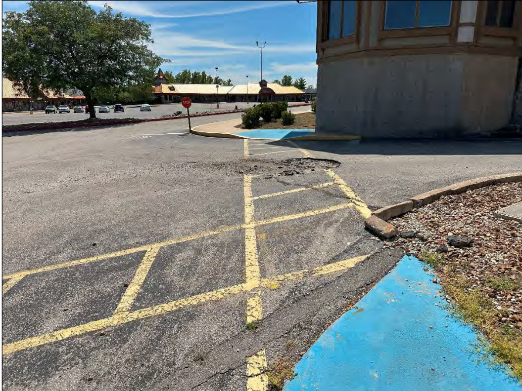
4540 Osage Beach Pkwy – deterioration of pavement
