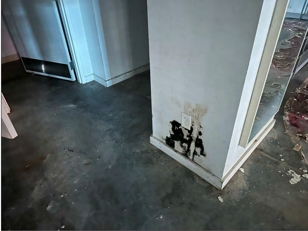
4540 Osage Beach Parkway – mold in retail space
