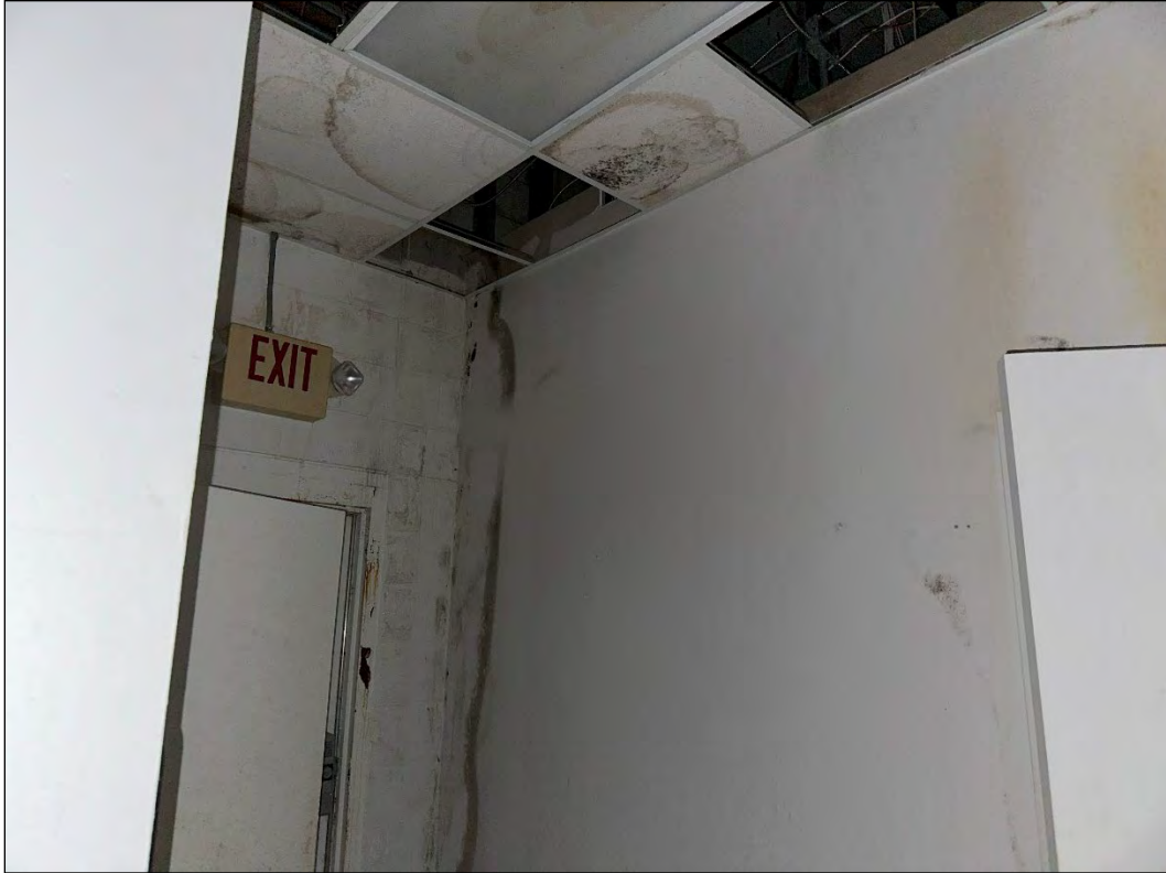
4540 Osage Beach Parkway – mold in retail space
