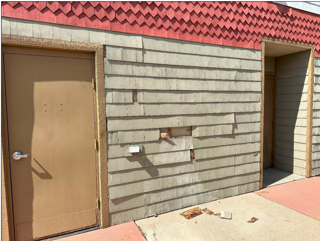
4540 Osage Beach Parkway – deterioration of wood siding; failure of finishes
