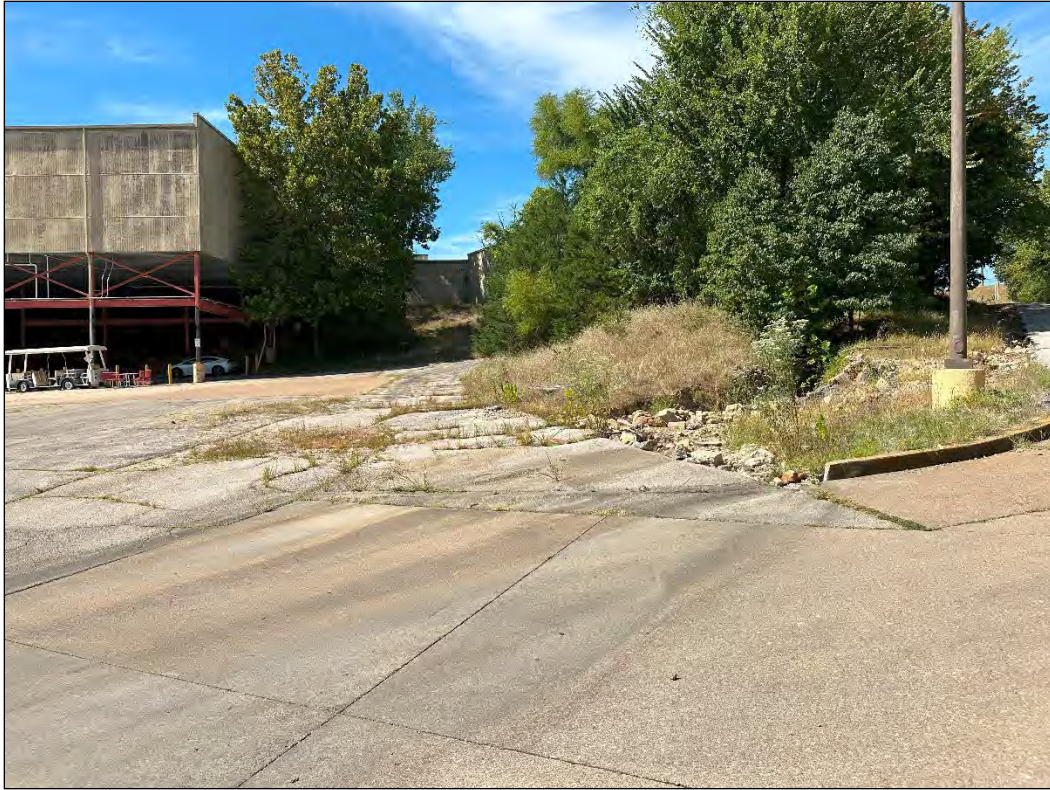
4540 Osage Beach Pkwy – deterioration of pavement
