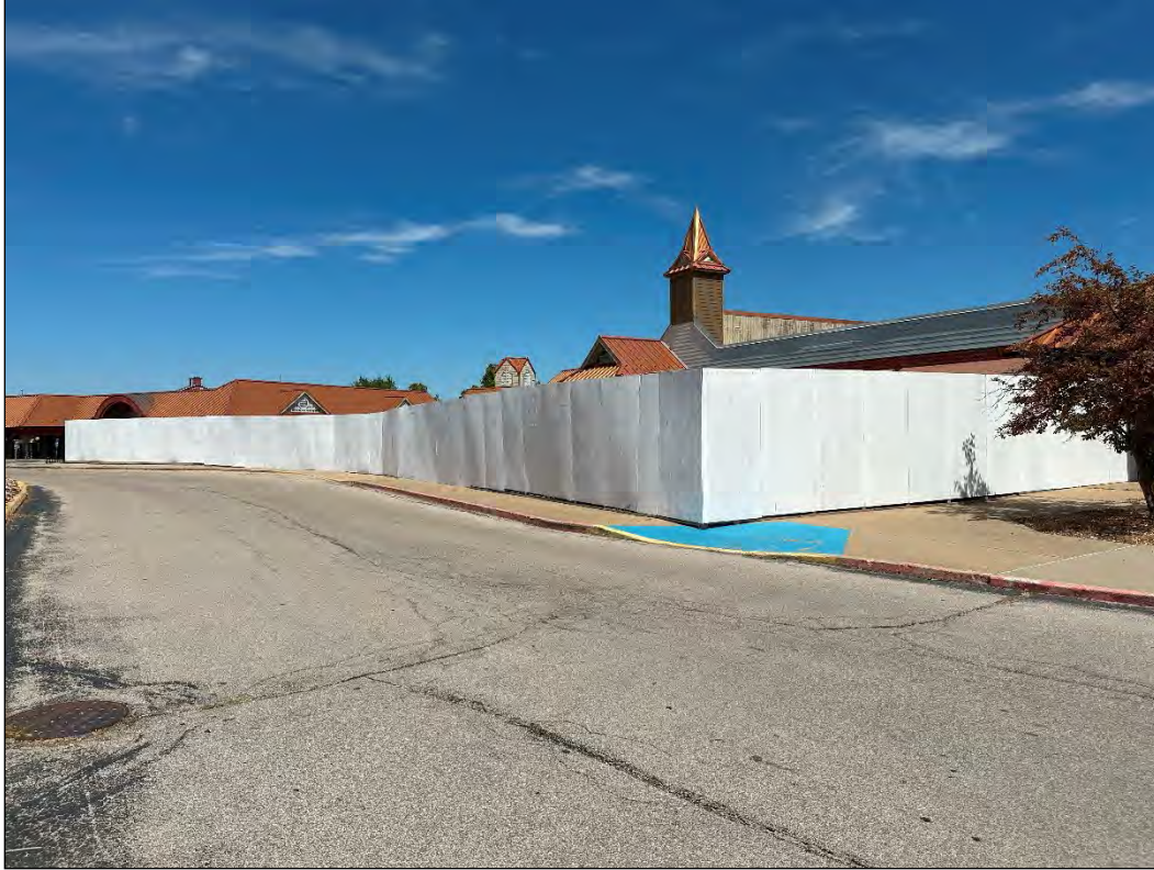
4540 Osage Beach Parkway – barricade preventing access to corroded steel walkways and stairs
