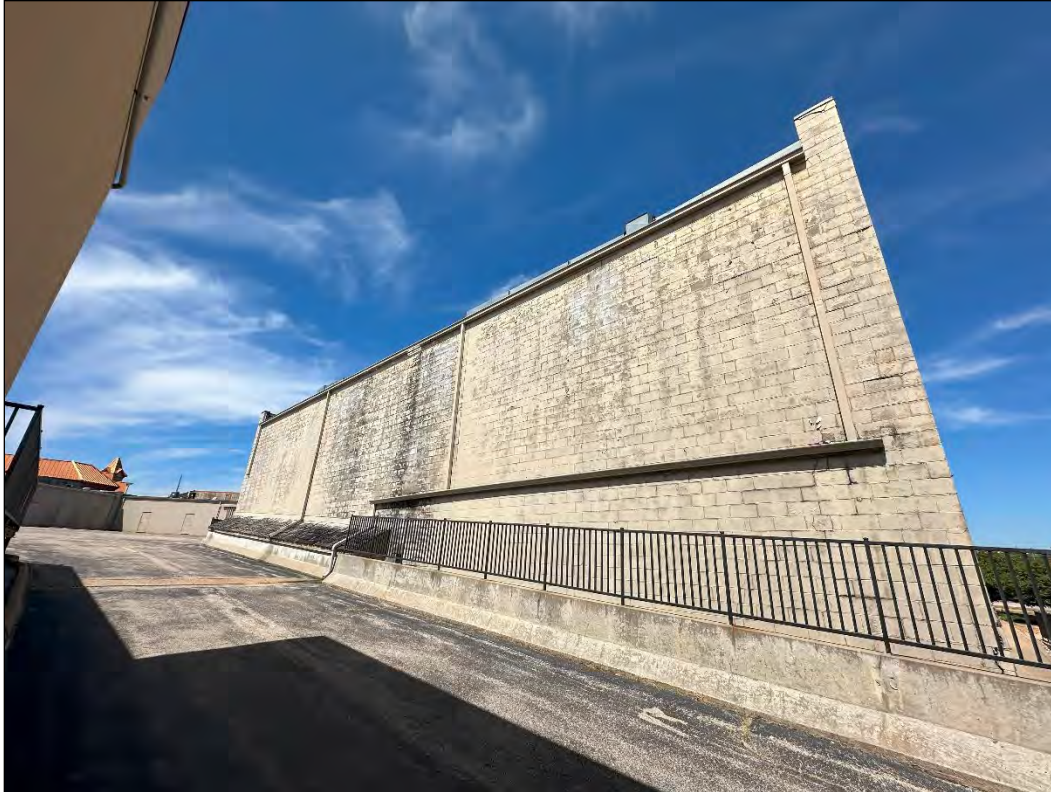
4540 Osage Beach Parkway – failure of finishes
