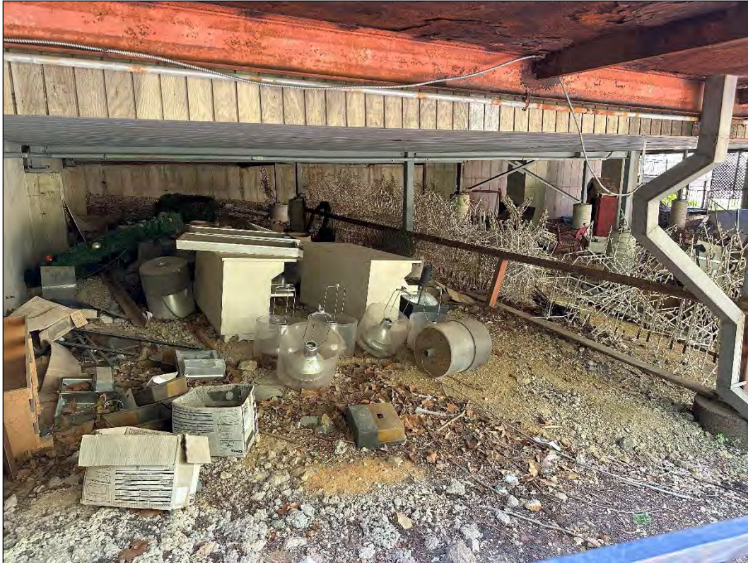
4540 Osage Beach Parkway – trash/debris
