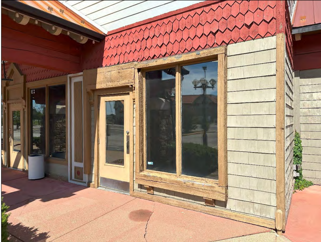
4540 Osage Beach Parkway – wood rot
