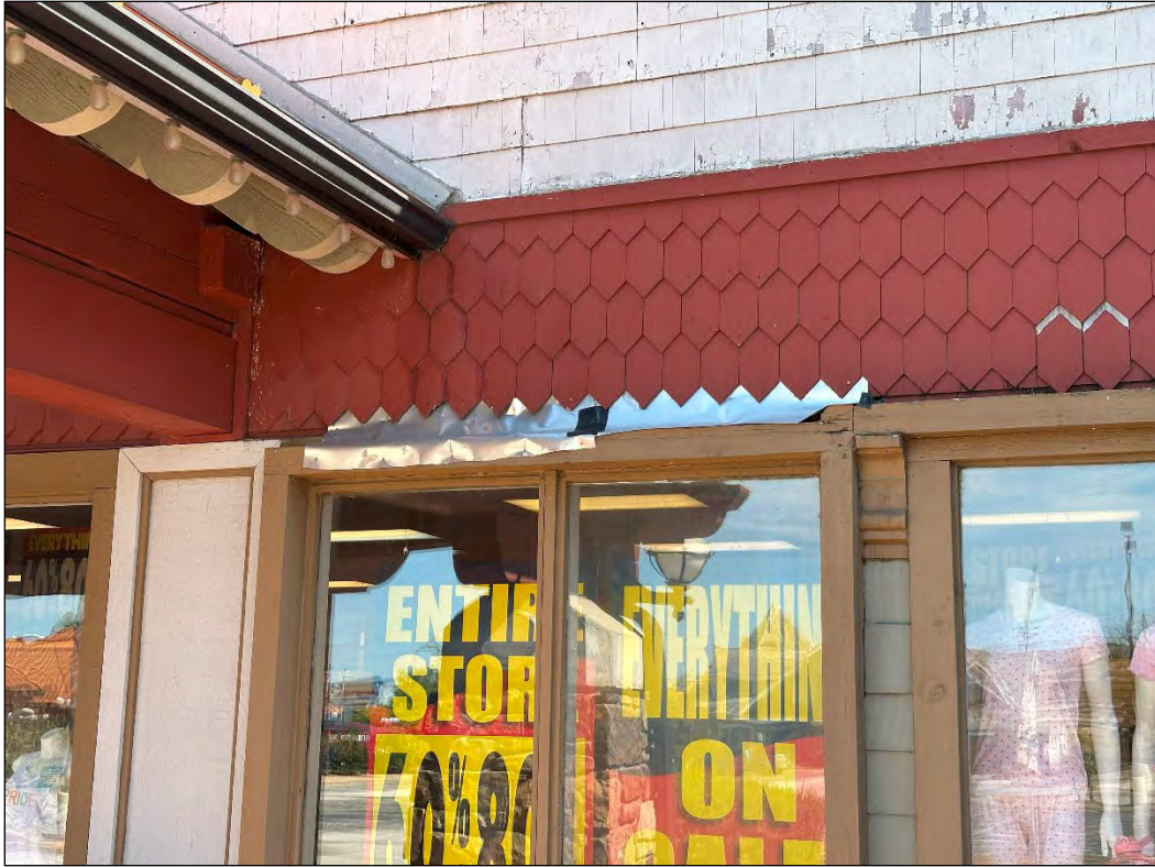
4540 Osage Beach Parkway – deterioration of flashing, wood siding and trim; failure of finishes
