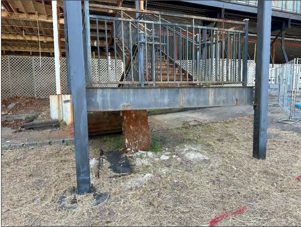
4540 Osage Beach Parkway – deterioration of steel stairs and landing; failure of finishes
