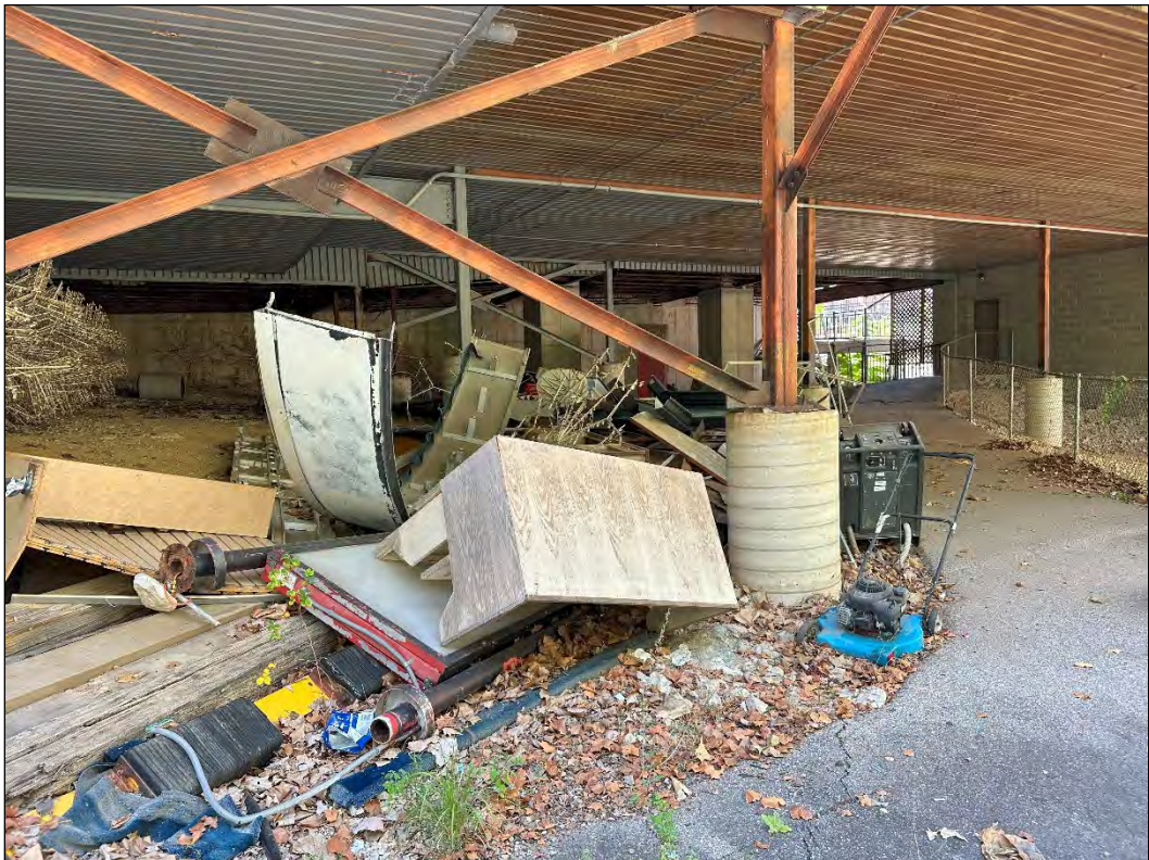
4540 Osage Beach Parkway – trash/debris
