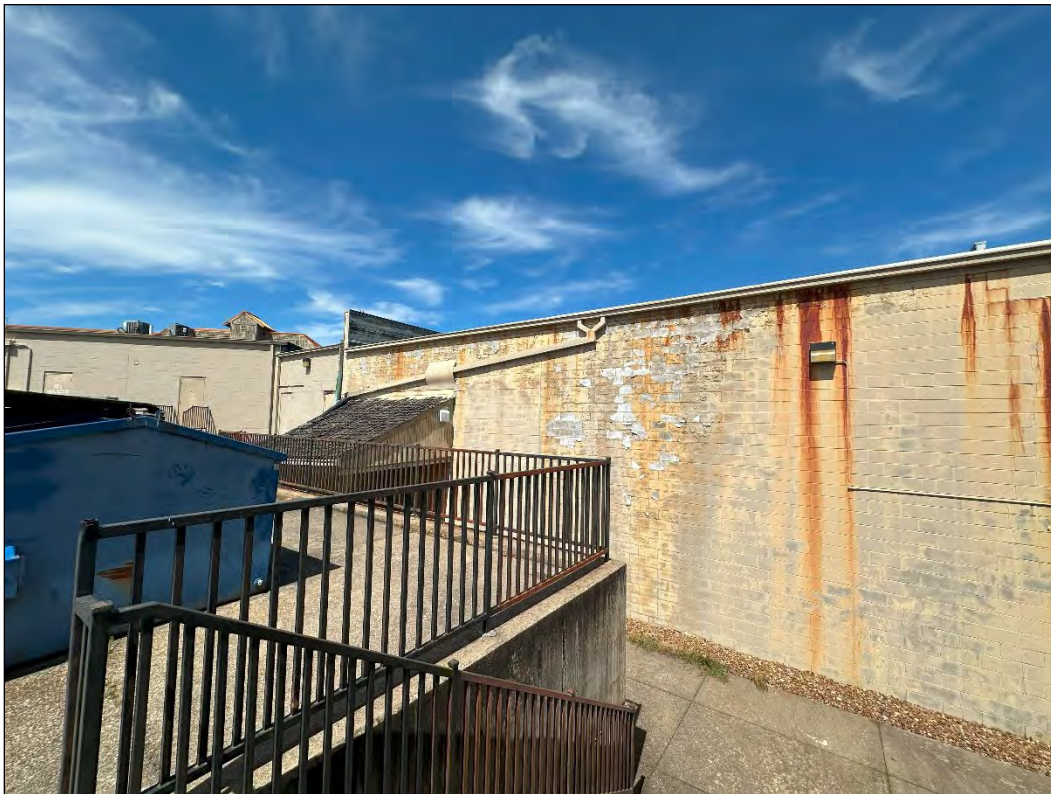
4540 Osage Beach Pkwy – failure of finishes; deterioration of gutters and downspouts
