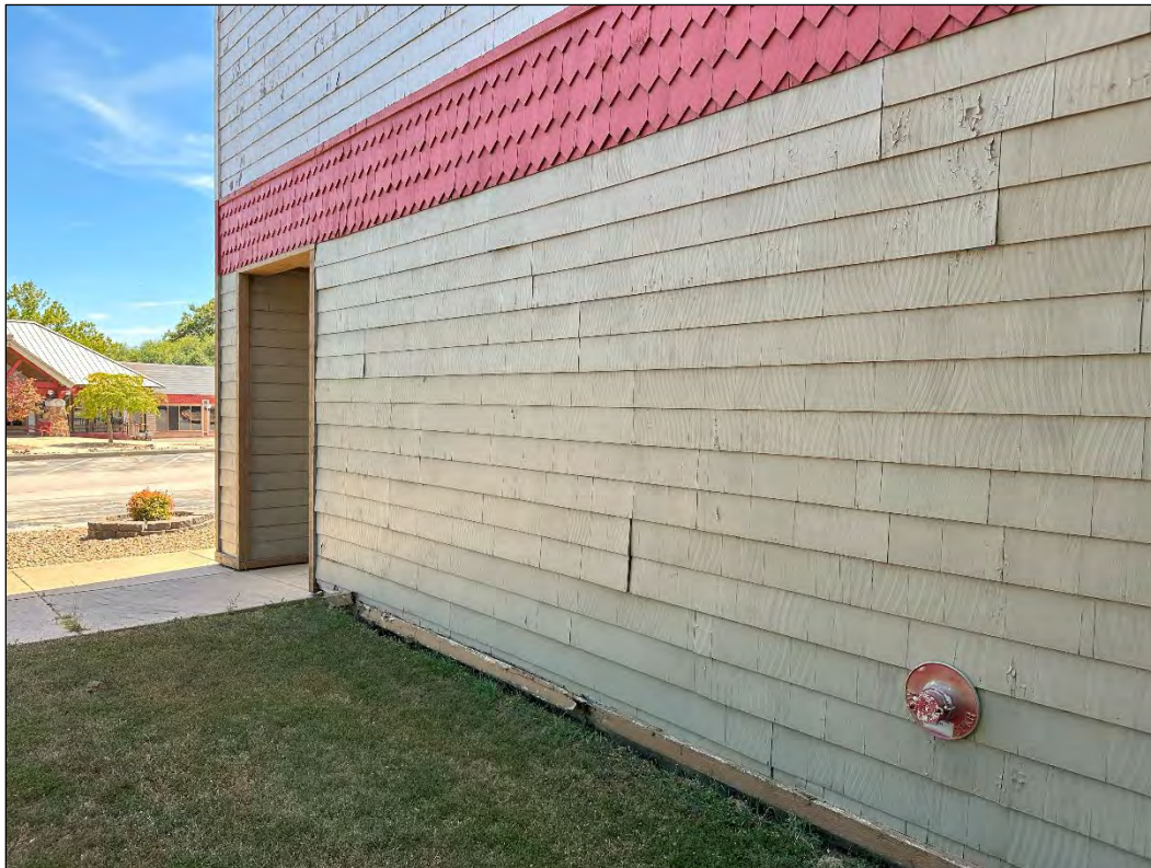
4540 Osage Beach Parkway – deterioration of wood siding, trim
