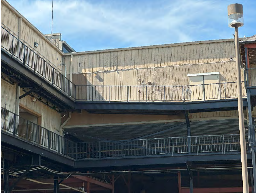
4540 Osage Beach Parkway – failure of finishes; deterioration of siding
