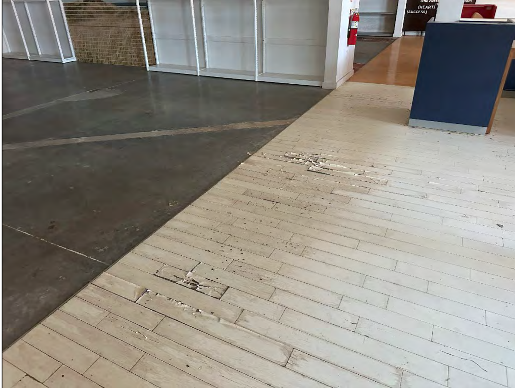
4540 Osage Beach Parkway – evidence of water damage caused by leaking roof/burst pipe
