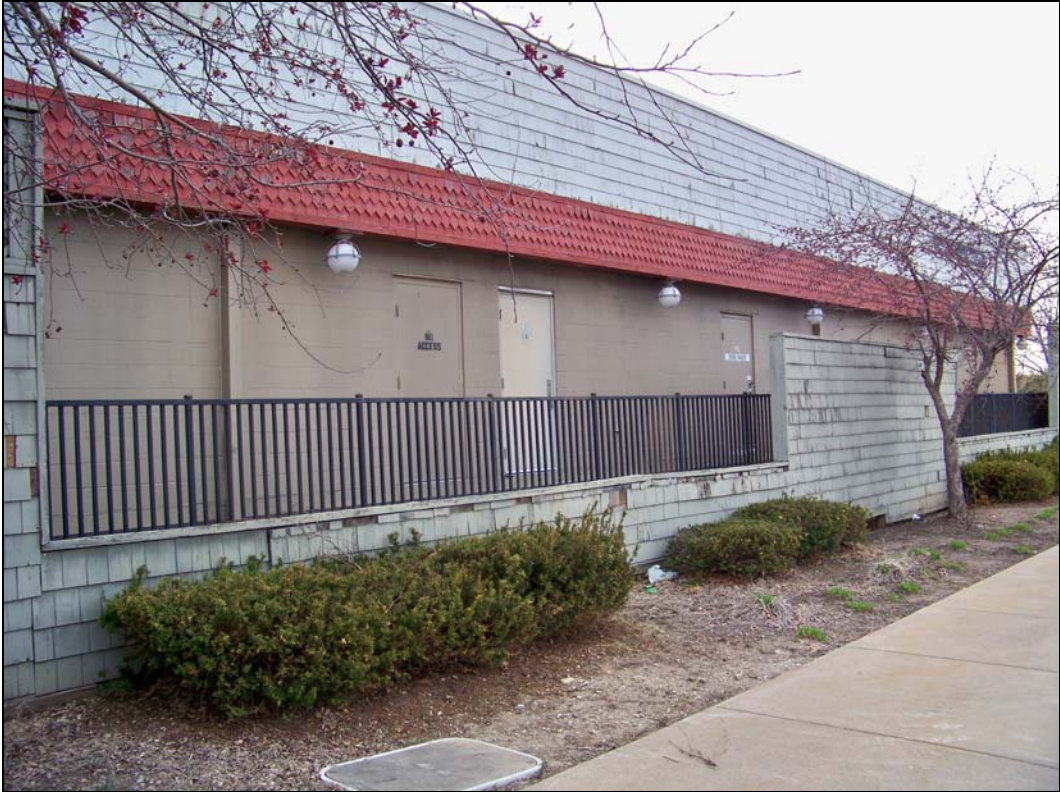
4540 Osage Beach Pkwy – looking southeast – deterioration of siding; failure of finishes
