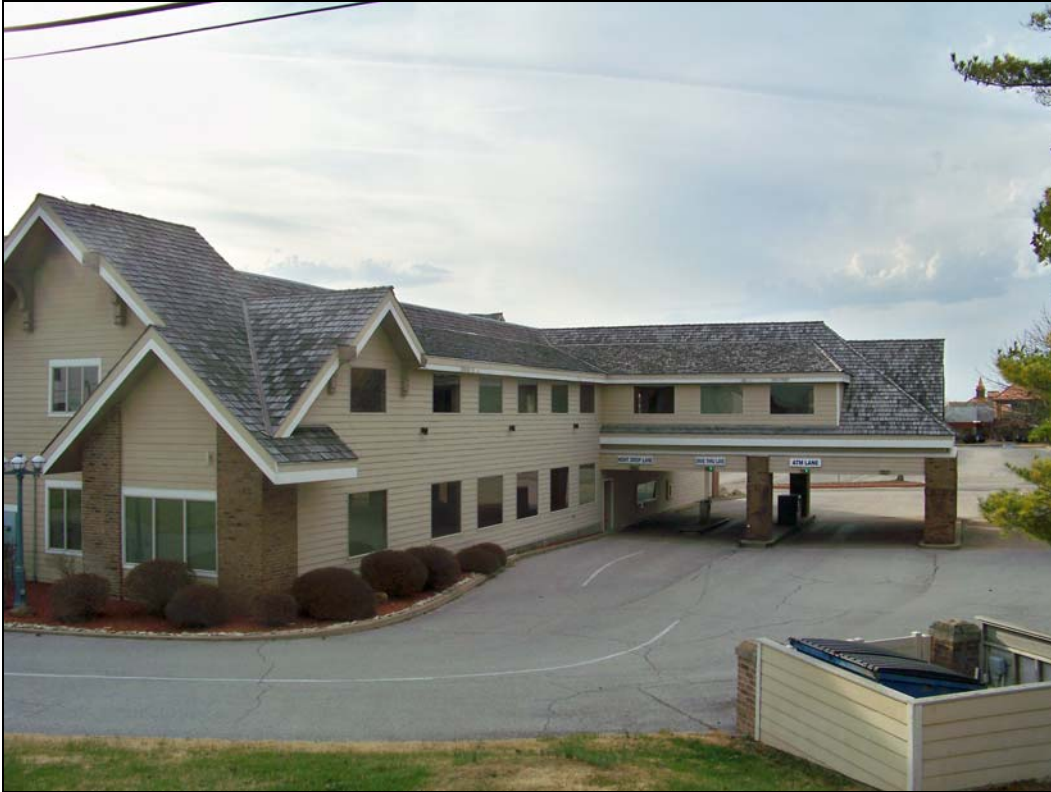
4558 Osage Beach Pkwy – looking south – deterioration of shake shingles, flashing; failure of finishes
