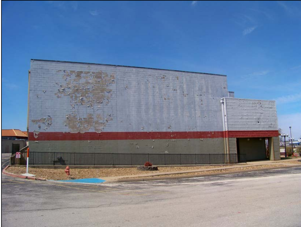
4540 Osage Beach Pkwy – looking west – failure of finishes
