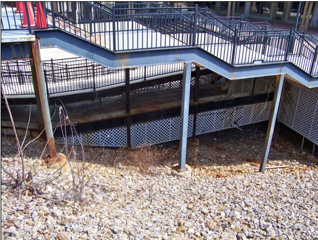
4540 Osage Beach Pkwy – looking east – deterioration of steel structure
