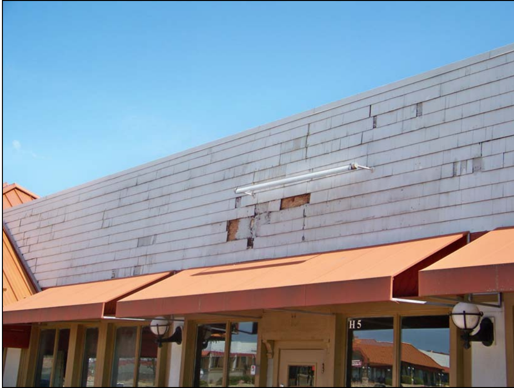
4540 Osage Beach Pkwy – looking northeast – deterioration of siding; failure of finishes
