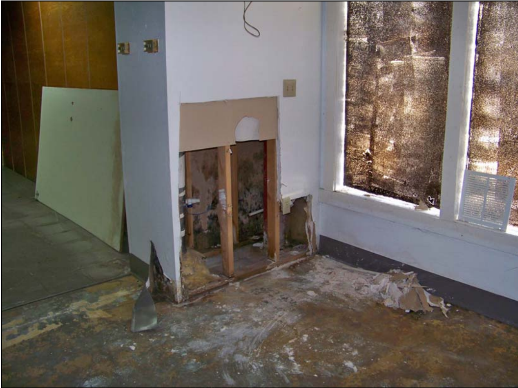
4540 Osage Beach Pkwy – interior – presence of mold
