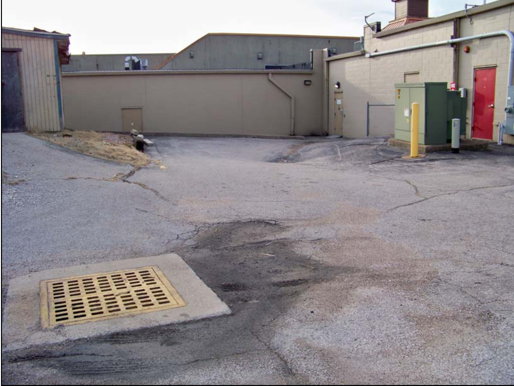
4540 Osage Beach Pkwy – looking east – deterioration of pavement
