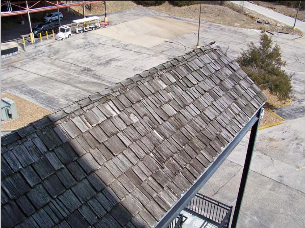
4540 Osage Beach Pkwy – looking east – deterioration of roof over stairs
