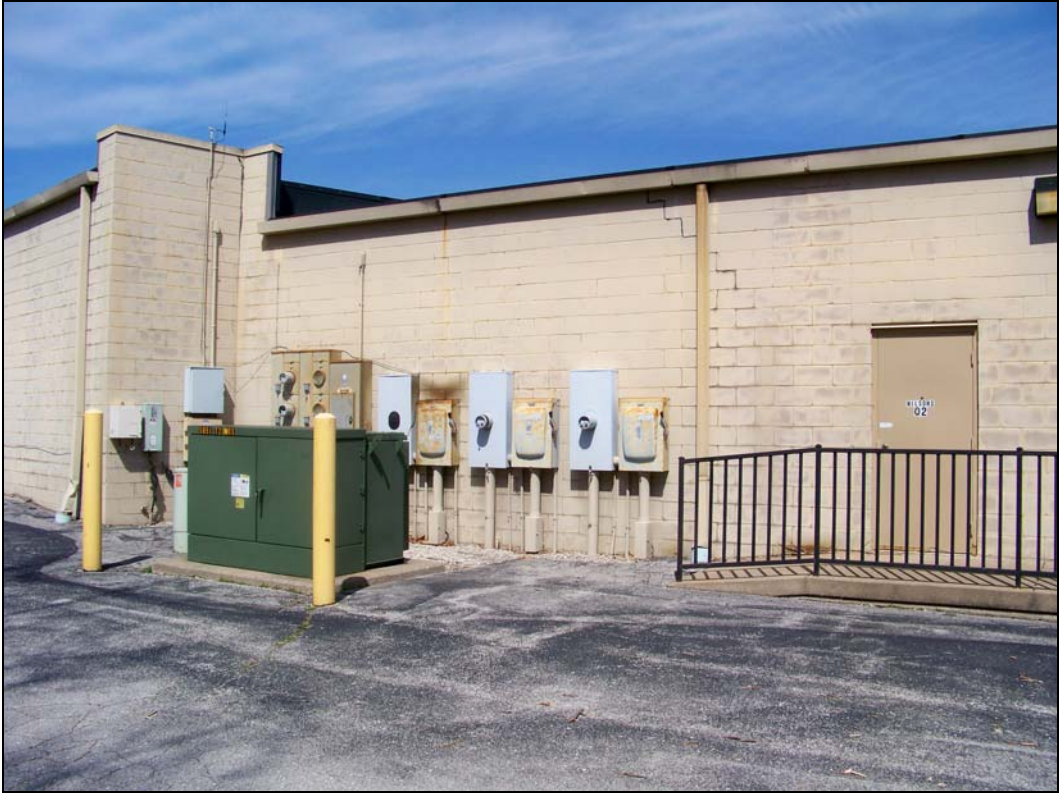
4540 Osage Beach Pkwy – looking north – failure of finishes; deterioration of equipment
