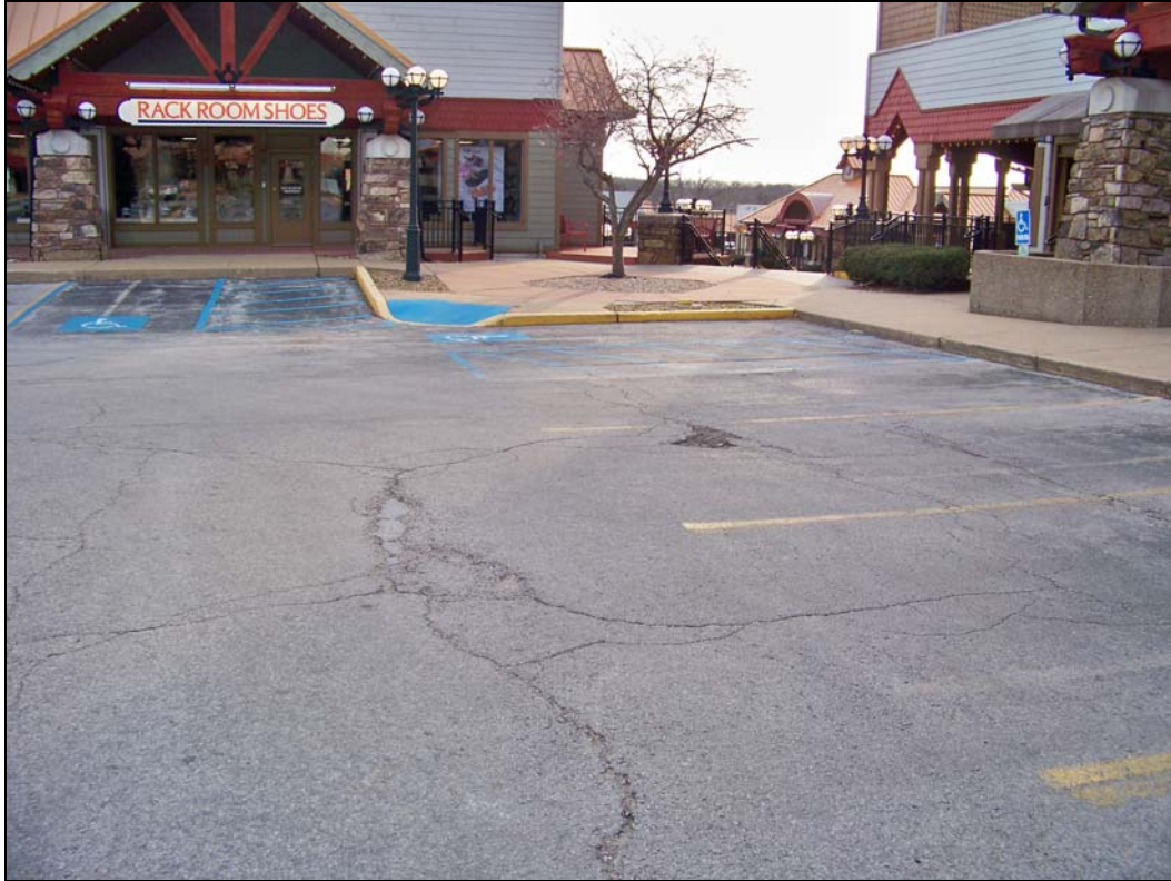
4540 Osage Beach Pkwy – looking south – lack of ADA signage and improper ADA sign (height)
