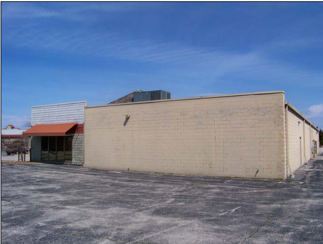
4540 Osage Beach Pkwy – looking north – failure of finishes
