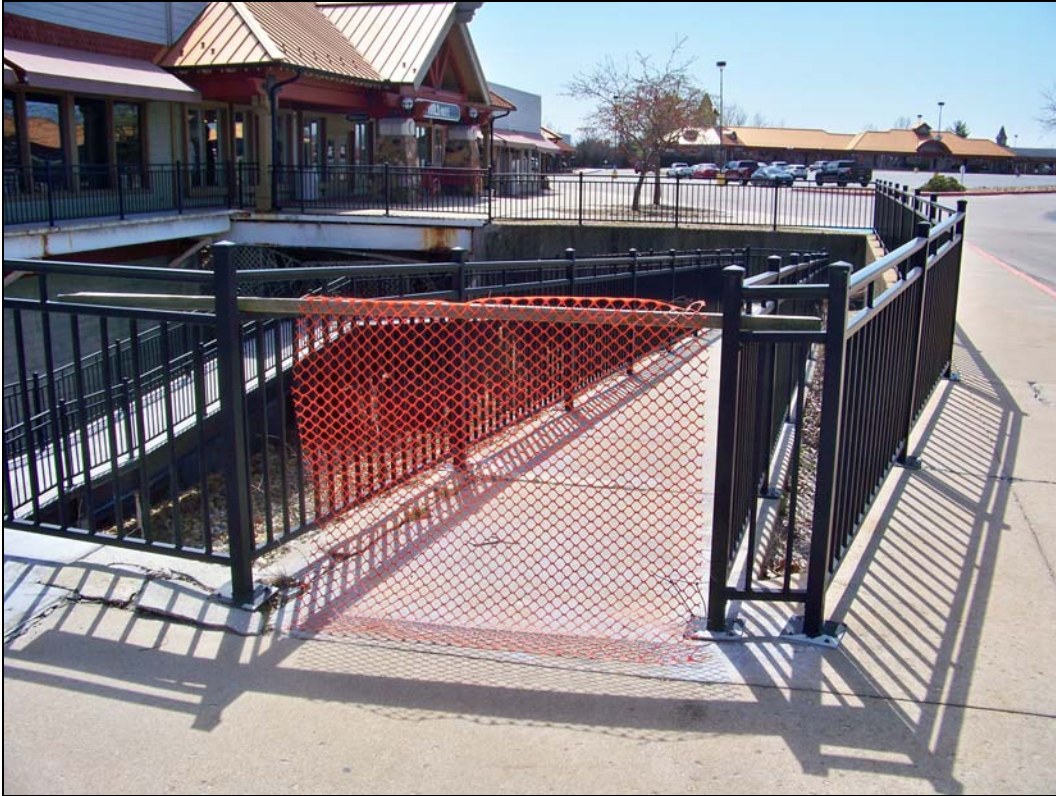
4540 Osage Beach Pkwy – looking south – walkway closure due to unsafe conditions (corroded steel)
