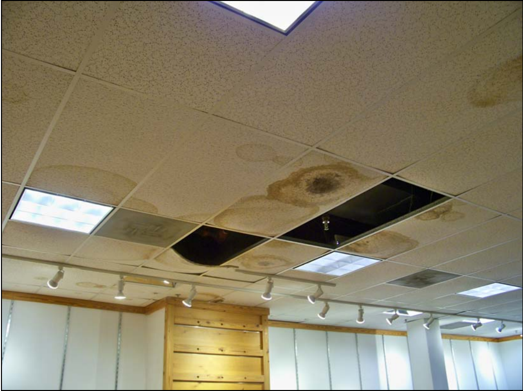
4540 Osage Beach Pkwy – interior – presence of mold
