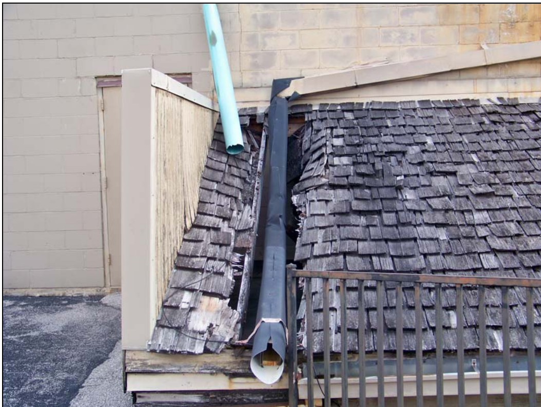
4540 Osage Beach Pkwy – looking west – deterioration of roof, fascia, downspouts; failure of finishes
