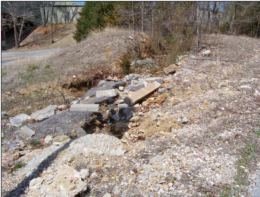
4540 Osage Beach Pkwy – looking north – trash/debris; poor drainage/erosion
