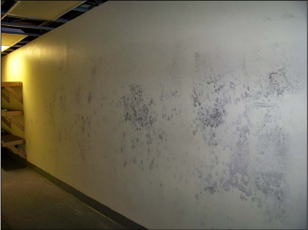
4540 Osage Beach Pkwy – interior – presence of mold
