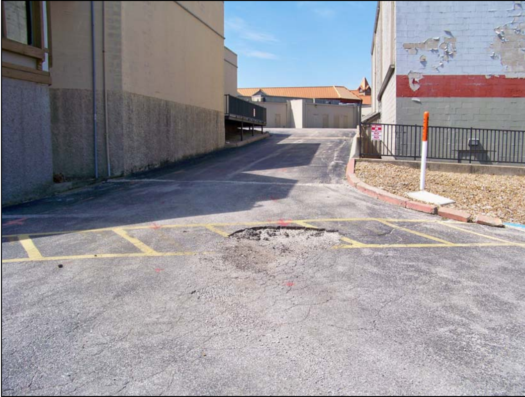
4540 Osage Beach Pkwy – looking west – deteriorated/uneven pedestrian crossing
