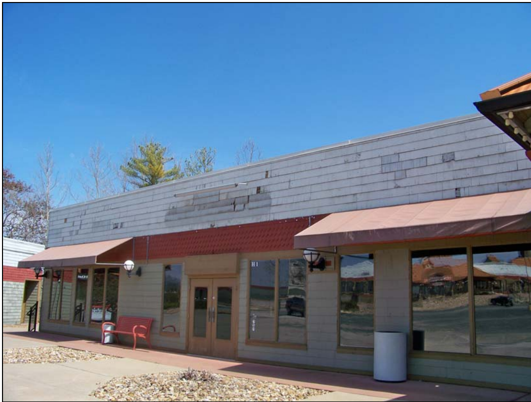
4540 Osage Beach Pkwy – looking east – deterioration of siding; failure of finishes
