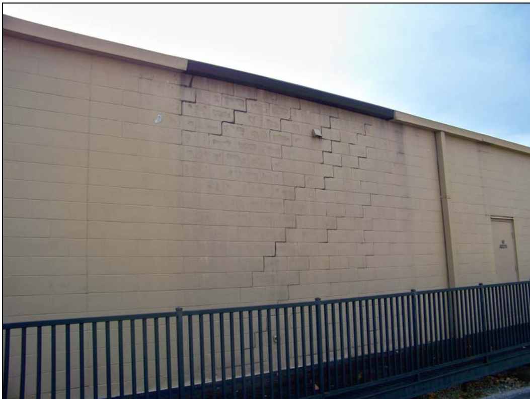
4540 Osage Beach Pkwy – looking east – deterioration of gutter, wall; failure of finishes
