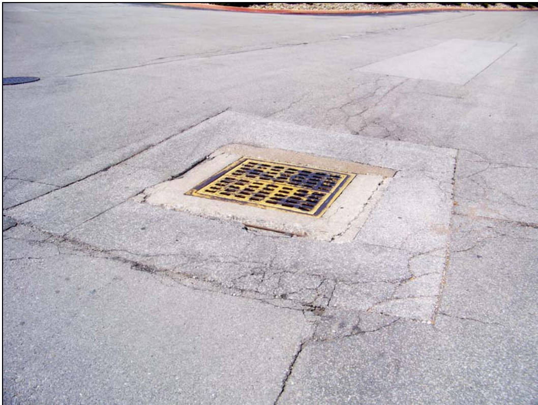
4540 Osage Beach Pkwy – looking north – deteriorated/uneven pavement/drain
