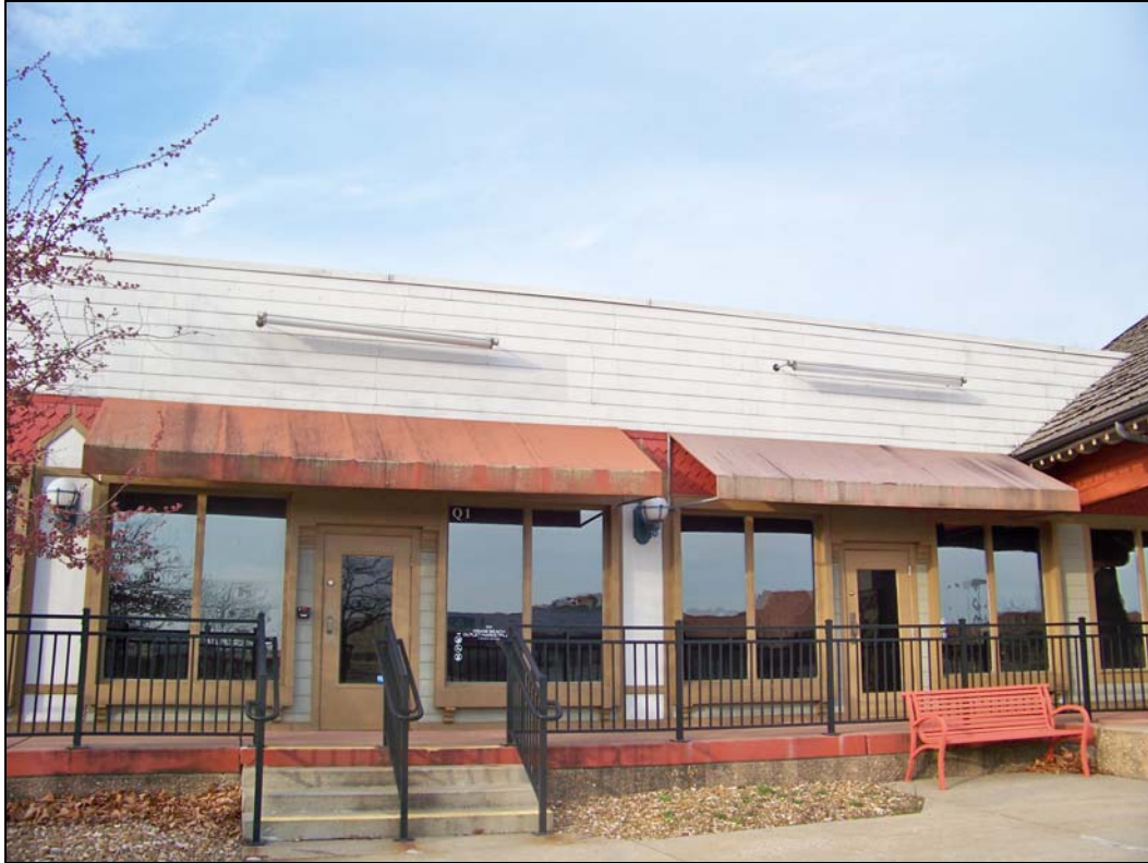
4540 Osage Beach Pkwy – looking west – deterioration of awnings
