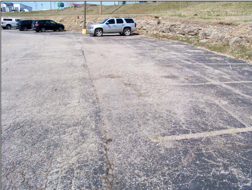
4540 Osage Beach Pkwy – looking northwest – deterioration of parking lot pavement
