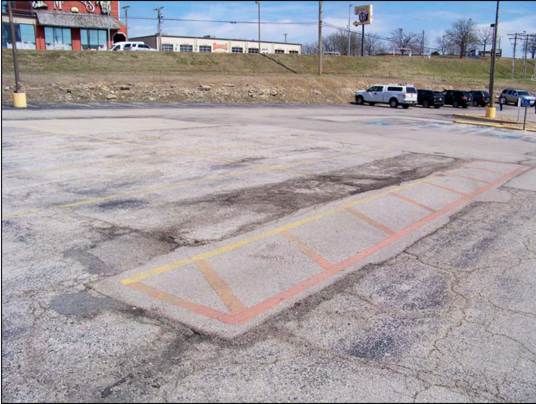
4540 Osage Beach Pkwy – looking northeast – deterioration of parking lot pavement
