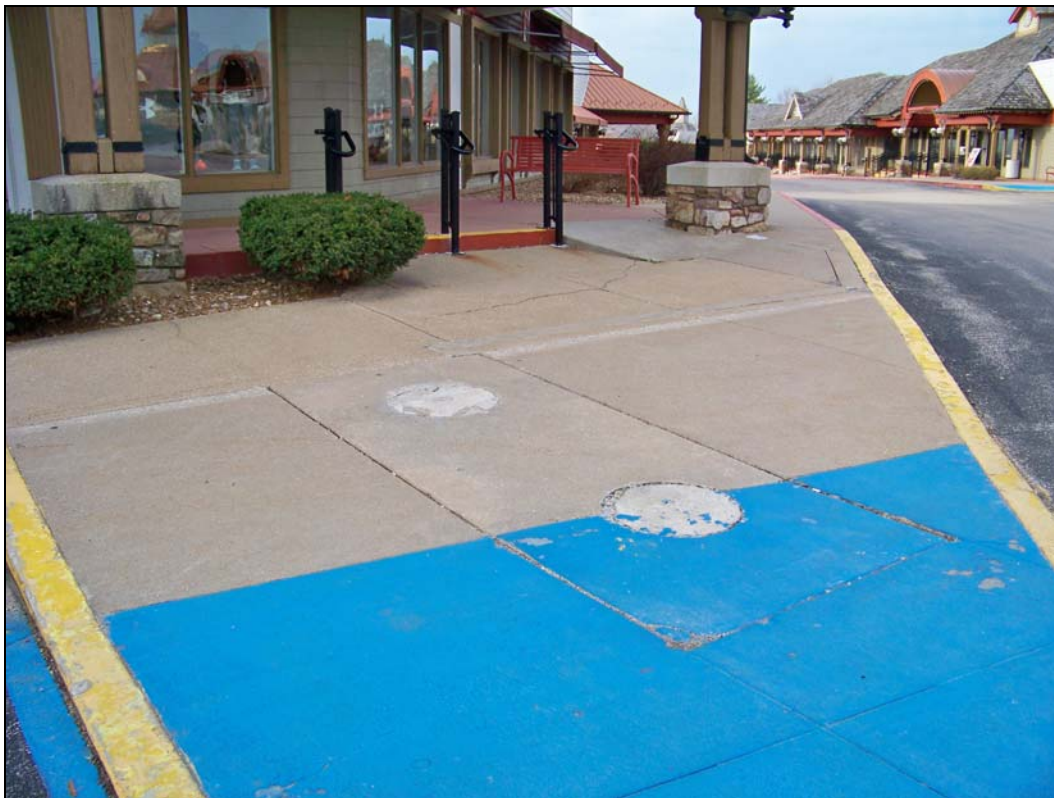
4540 Osage Beach Pkwy – looking south – improper ramp per ADA code
