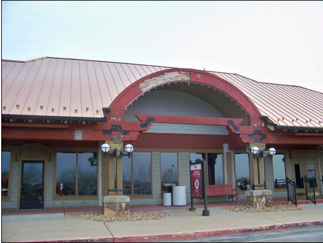
4540 Osage Beach Pkwy – looking north – deterioration of trim
