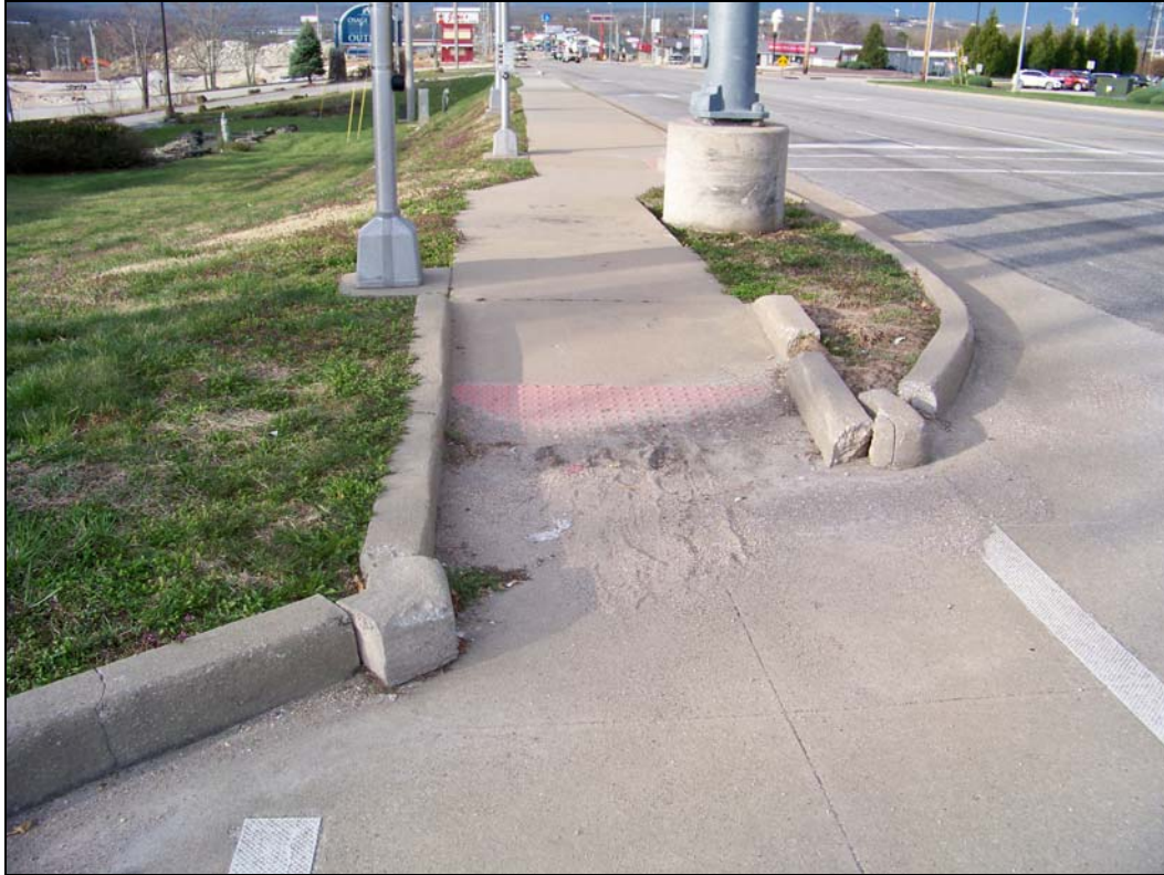
4644 Osage Beach Pkwy – looking south – debris-covered sidewalk; deterioration of curb
