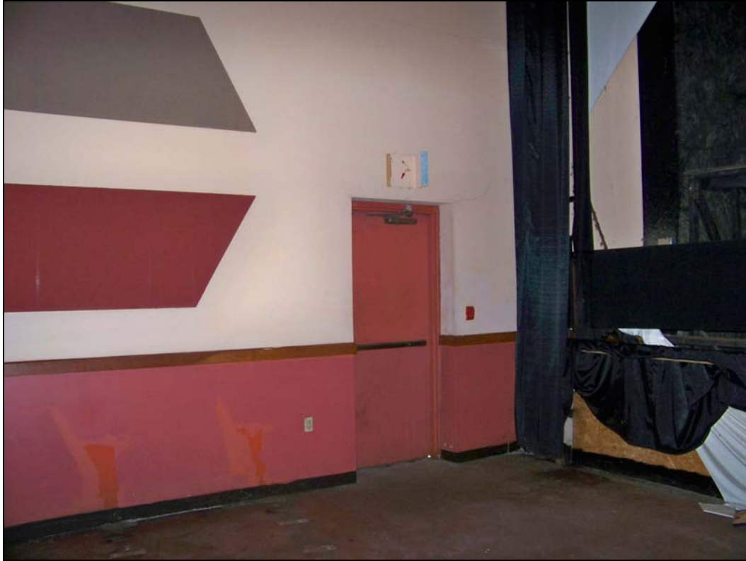
4540 Osage Beach Pkwy – interior – lack of emergency signage
