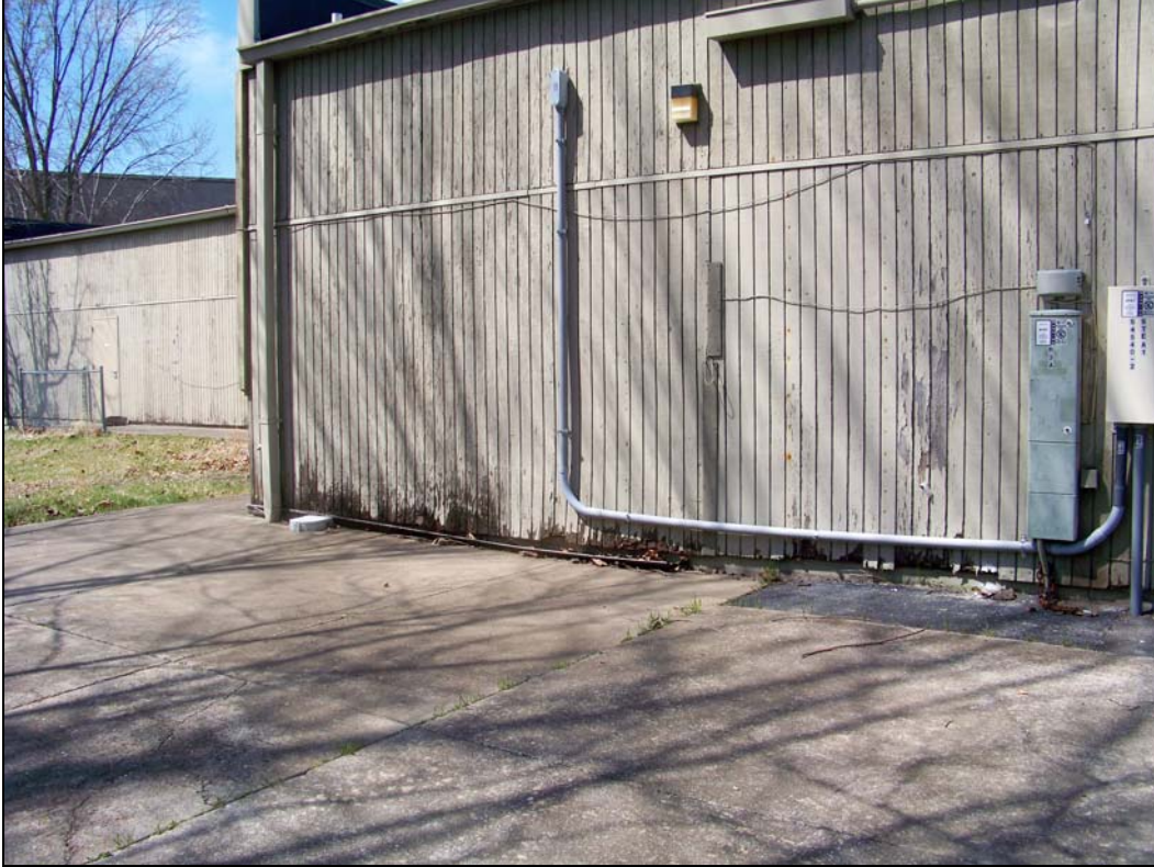
4540 Osage Beach Pkwy – looking west – deterioration of siding; failure of finishes
