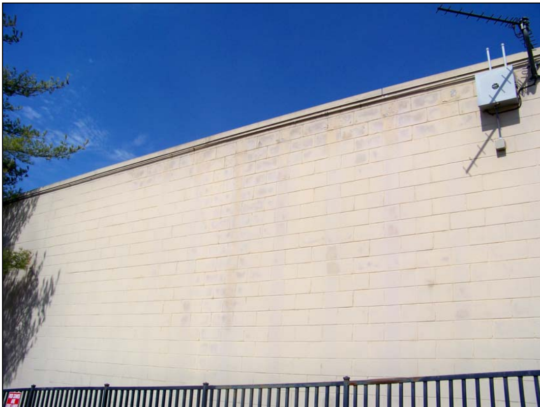
4540 Osage Beach Pkwy – looking east – failure of finishes
