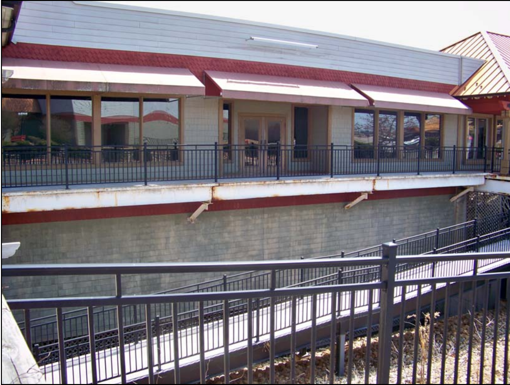
4540 Osage Beach Pkwy – looking east – deterioration of steel structure; failure of finishes
