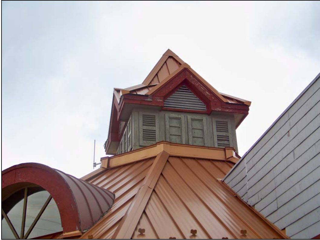
4540 Osage Beach Pkwy – looking south – deterioration of siding; failure of finishes
