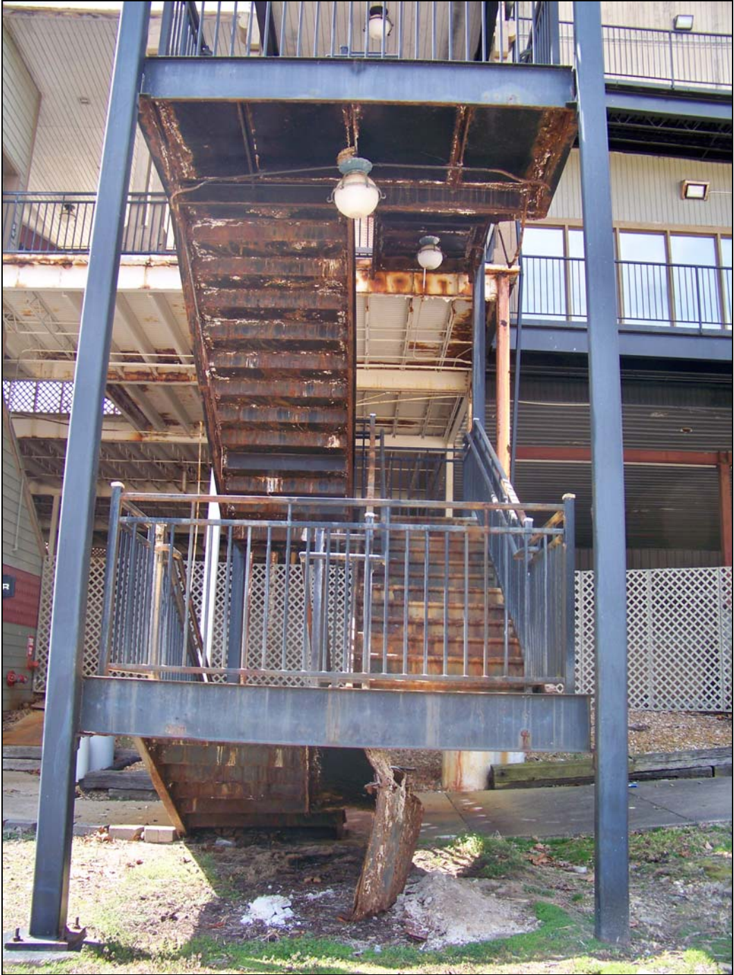
4540 Osage Beach Pkwy – looking west – closure of stairs due to corroded steel structure, collapse of landing
