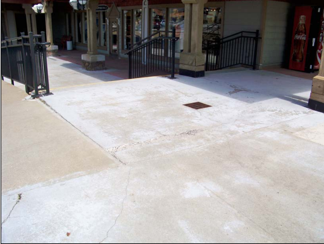
4540 Osage Beach Pkwy – looking east – deteriorated/uneven pedestrian walkway
