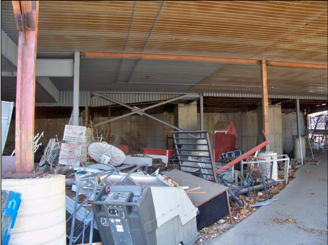
4540 Osage Beach Pkwy – looking west – trash/debris
