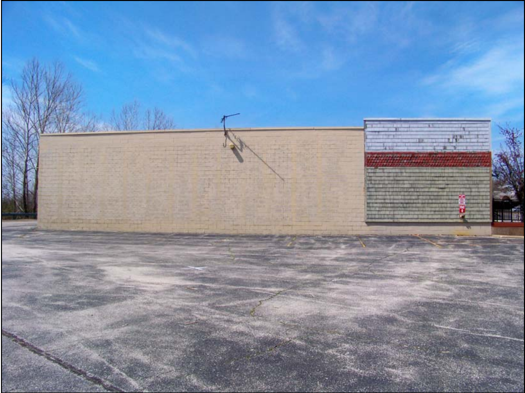
4540 Osage Beach Pkwy – looking northwest – deterioration of siding; failure of finishes
