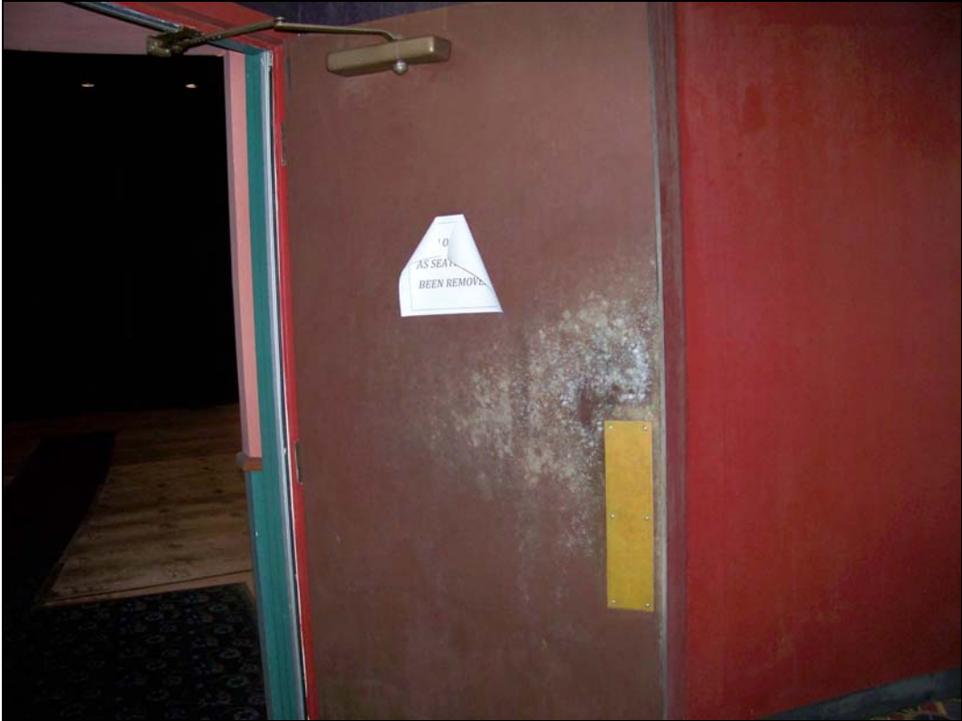
4540 Osage Beach Pkwy – interior – presence of mold
