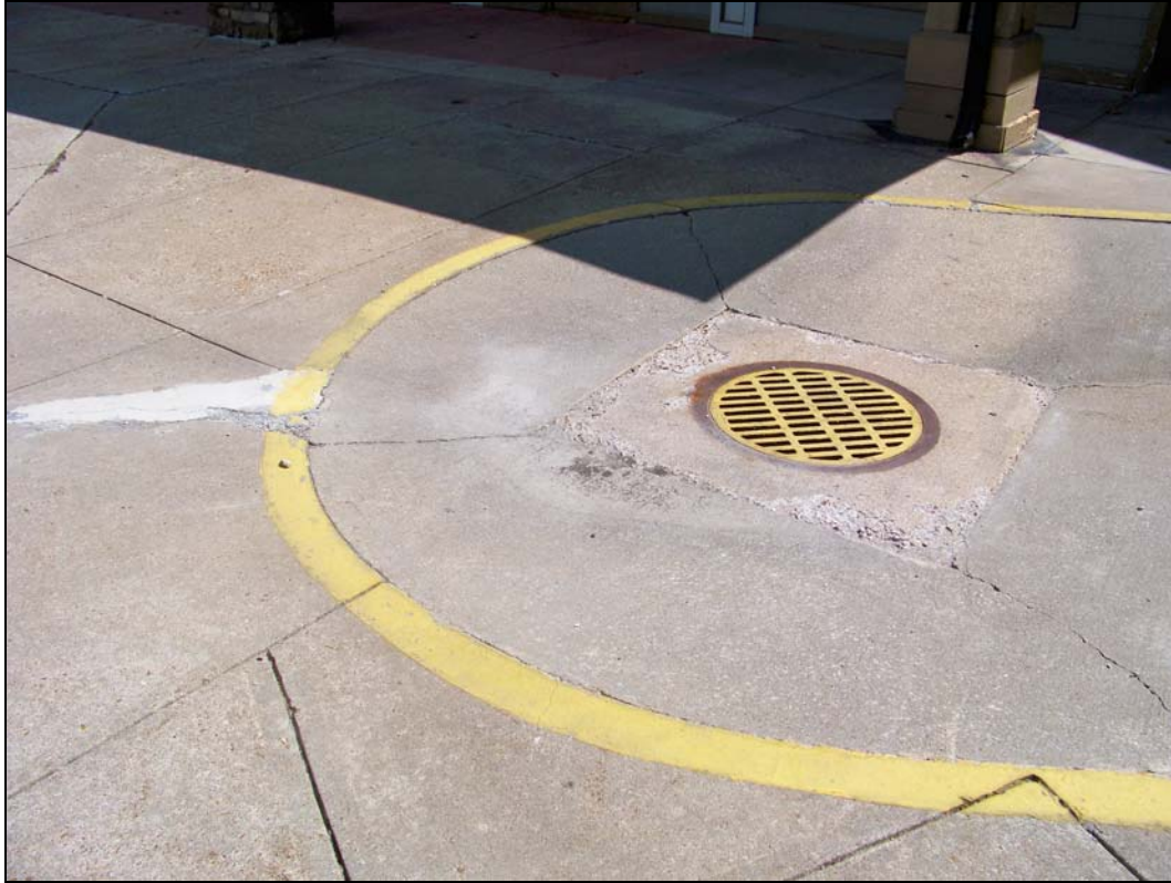
4540 Osage Beach Pkwy – looking east – deteriorated/uneven pavement/drain
