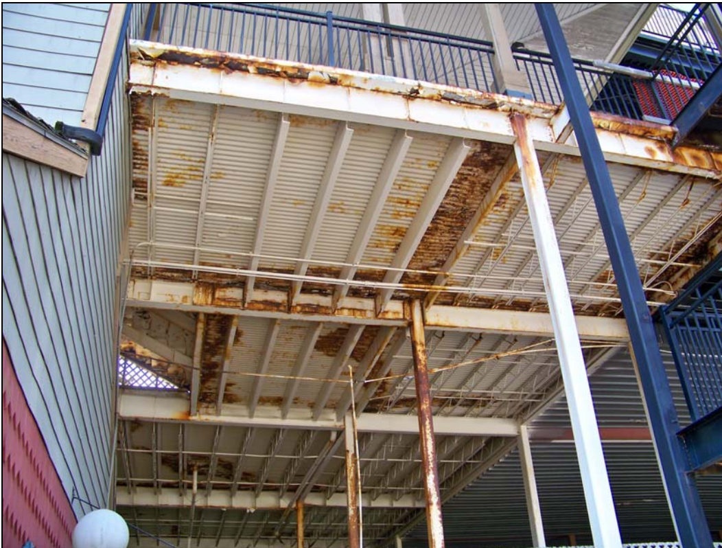
4540 Osage Beach Pkwy – looking west – deterioration of steel structure; failure of finishes
