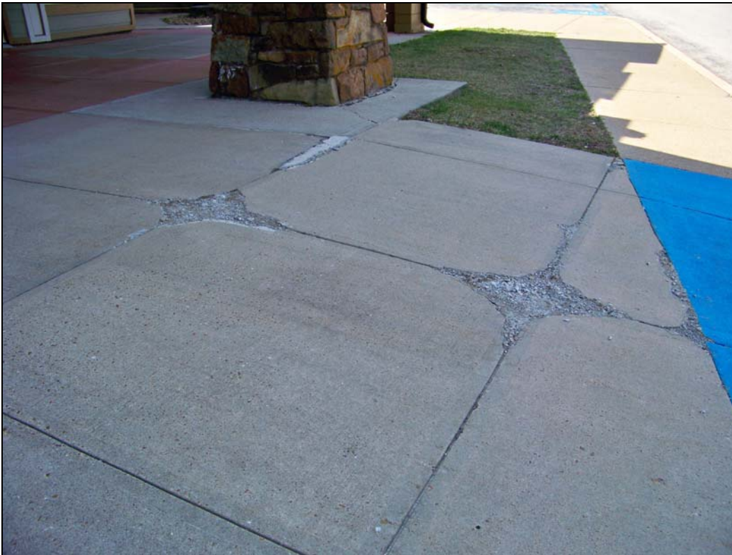
4540 Osage Beach Pkwy – looking north – deteriorated/uneven pedestrian walkway
