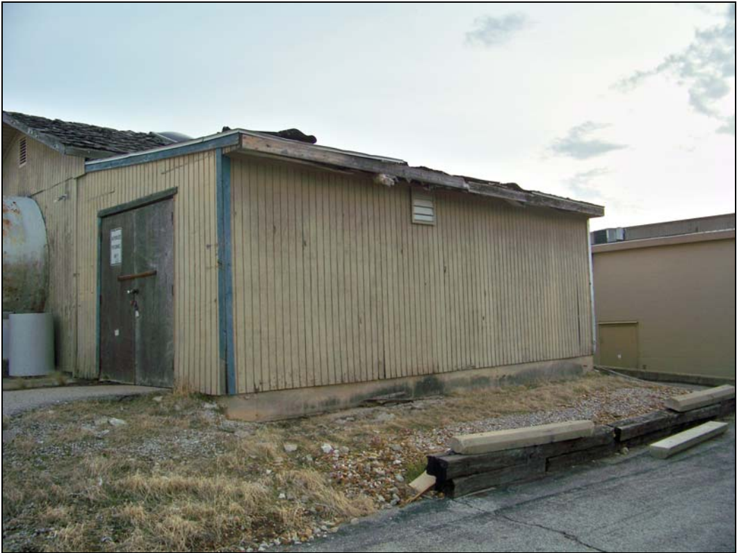
4540 Osage Beach Pkwy – looking north – deterioration of ancillary structure
