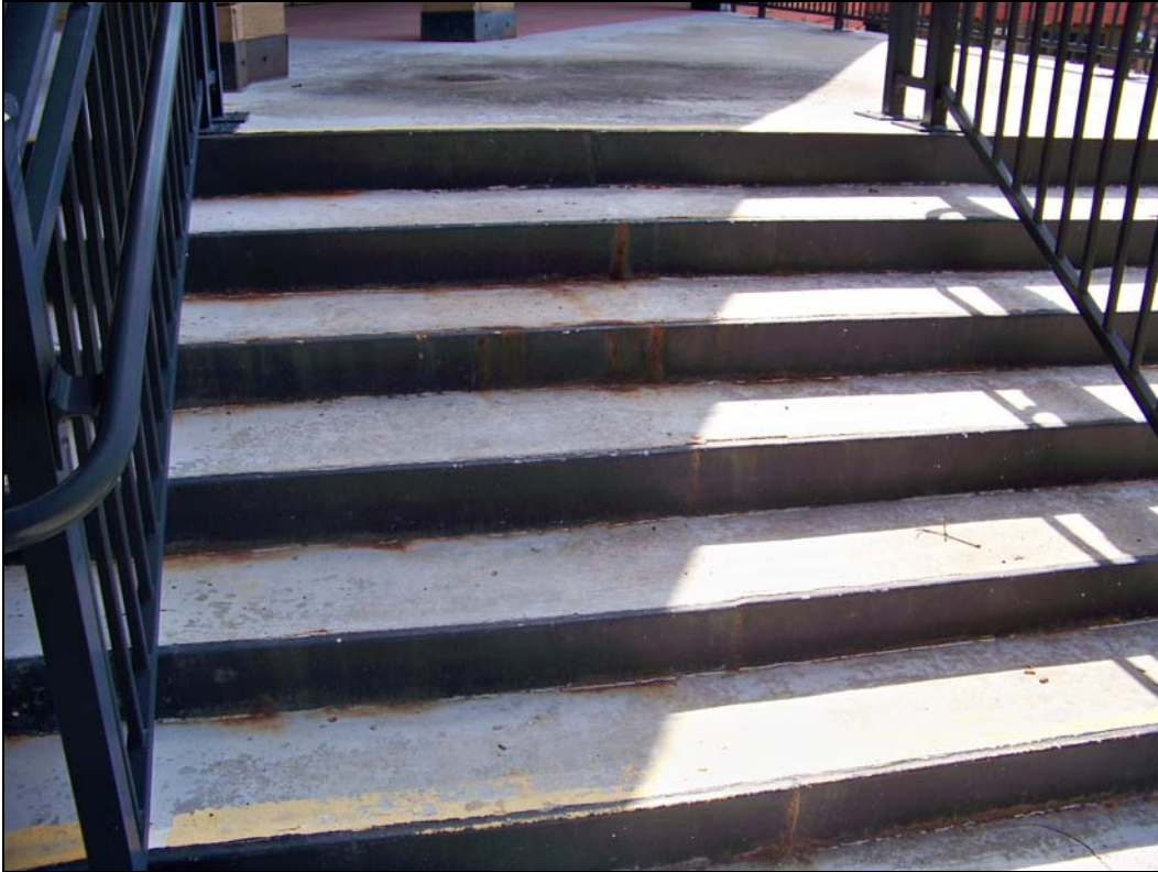
4540 Osage Beach Pkwy – looking east – deterioration of stairs
