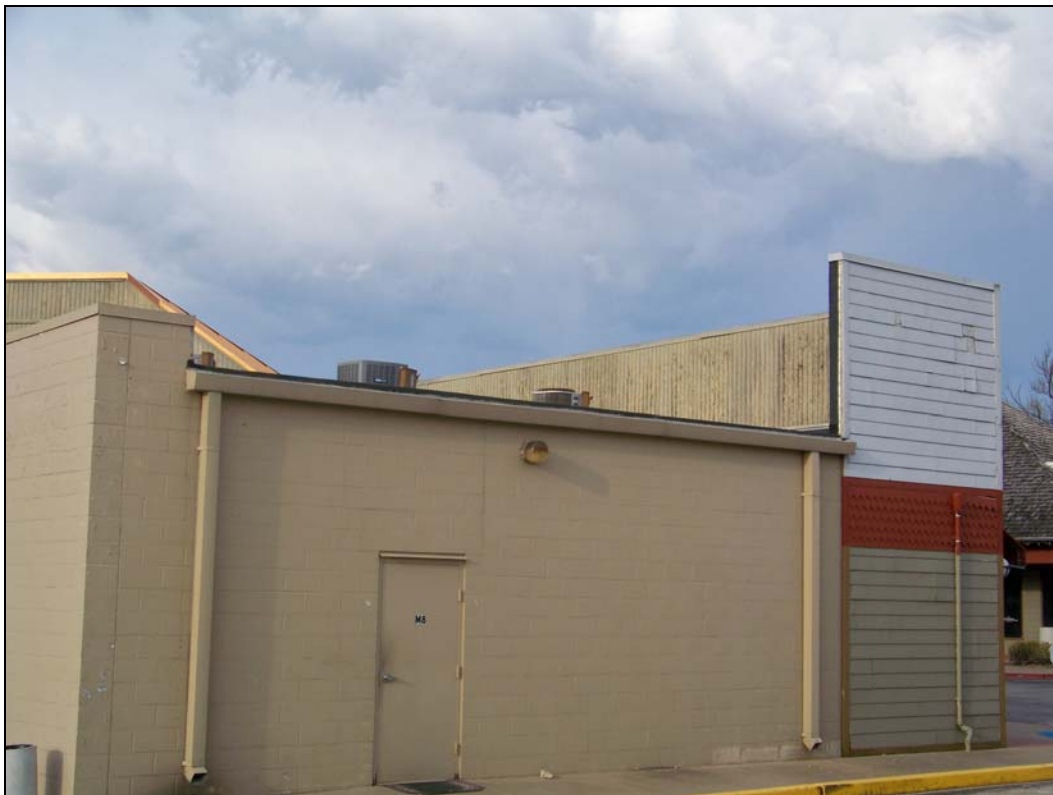
4540 Osage Beach Pkwy – looking south – deterioration of siding, parapet wall; failure of finishes
