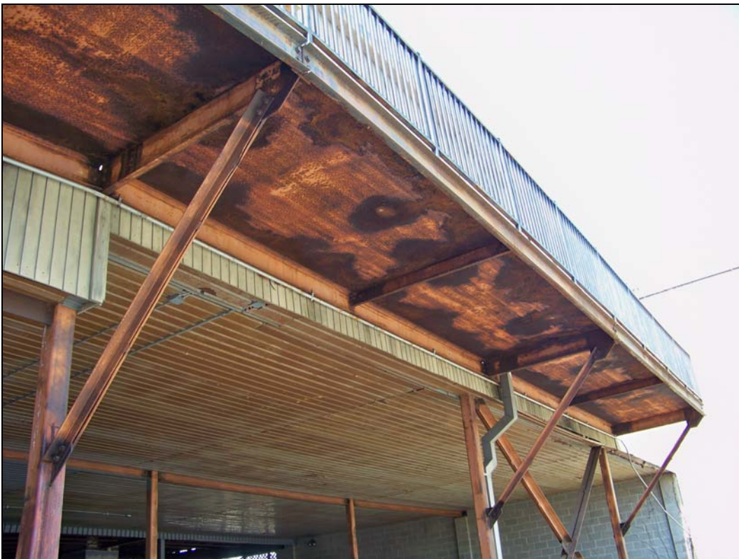
4540 Osage Beach Pkwy – looking west – corroded steel structure and walkway
