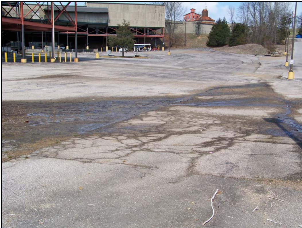
4540 Osage Beach Pkwy – looking north – deterioration of parking lot pavement
