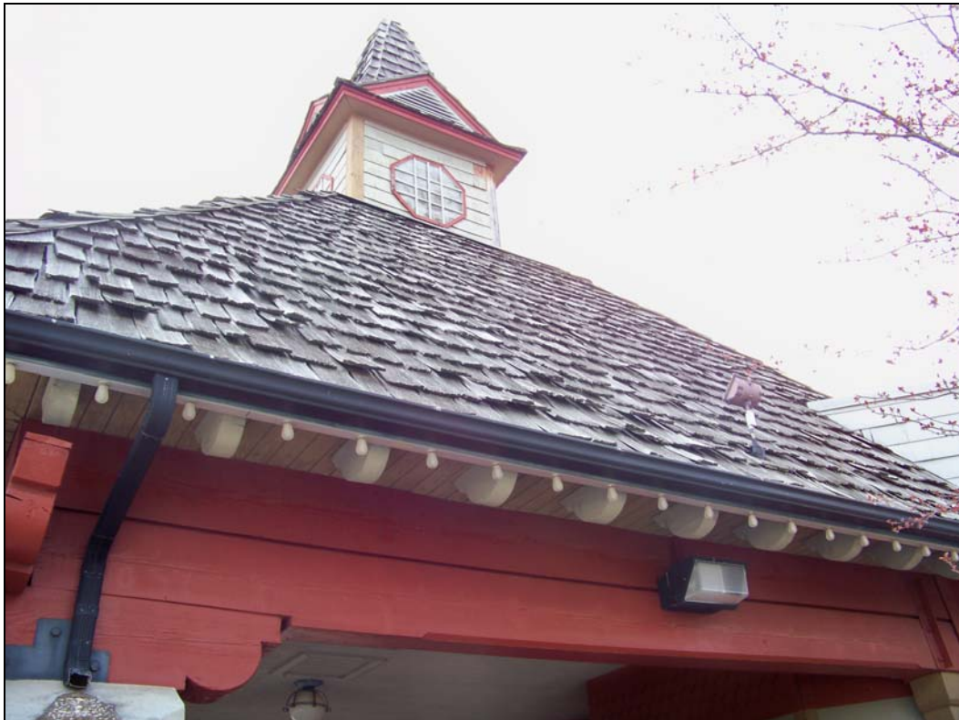
4540 Osage Beach Pkwy – looking south – deterioration of shake shingles, siding; failure of finishes
