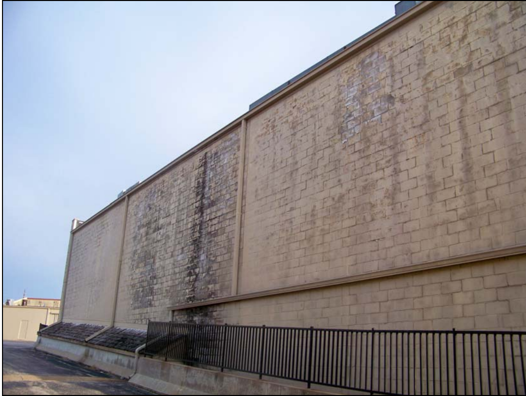
4540 Osage Beach Pkwy – looking northwest – deterioration of shake shingles; failure of finishes
