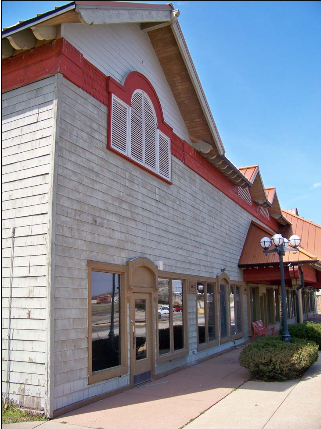
4540 Osage Beach Pkwy – looking northwest – deterioration of siding; failure of finishes
