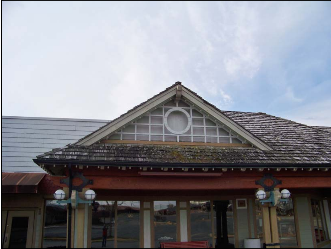
4540 Osage Beach Pkwy – looking south – deterioration of shake shingle roof, siding
