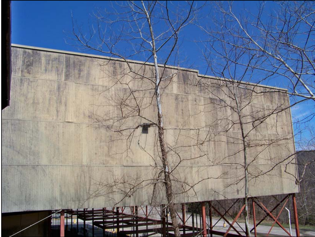
4540 Osage Beach Pkwy – looking north – deterioration of siding; failure of finishes
