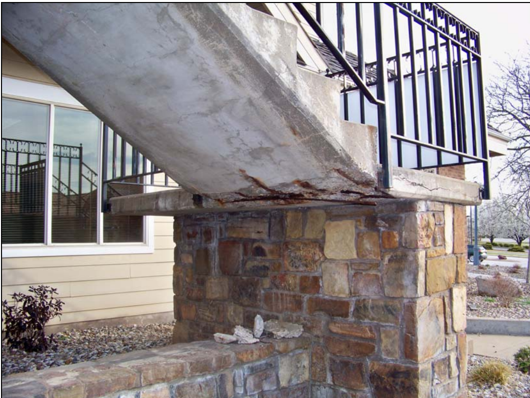
4540 Osage Beach Pkwy – looking northeast – deterioration of stairs
