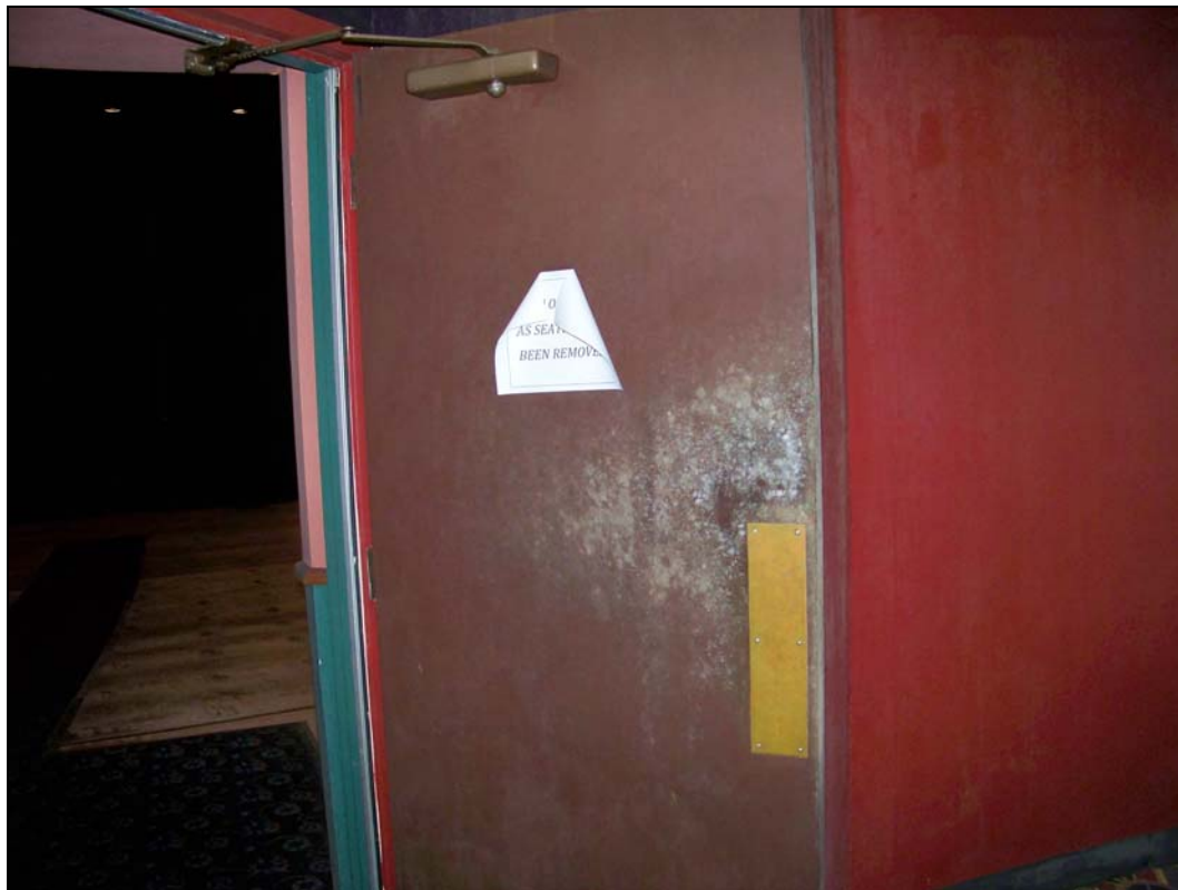
4540 Osage Beach Pkwy – interior – presence of mold
