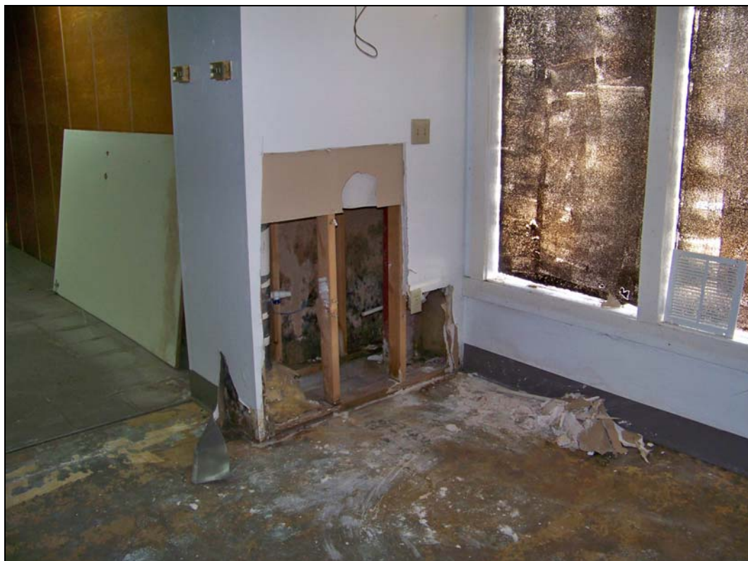
4540 Osage Beach Pkwy – interior – presence of mold
