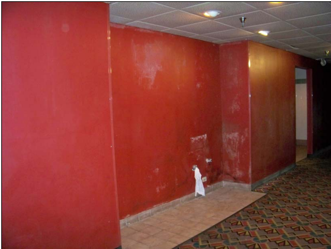
4540 Osage Beach Pkwy – interior – presence of mold
