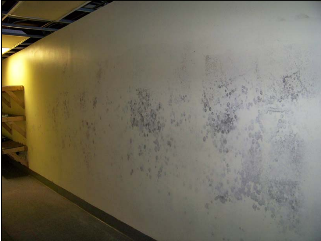
4540 Osage Beach Pkwy – interior – presence of mold
