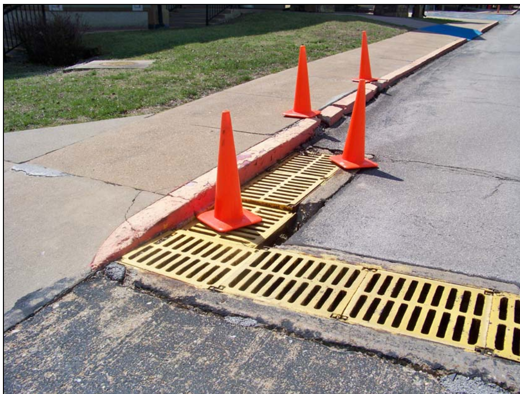
4540 Osage Beach Pkwy – looking southwest – deteriorated/uneven pavement/drain
