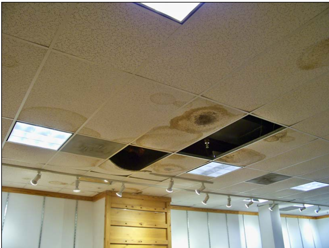
4540 Osage Beach Pkwy – interior – presence of mold
