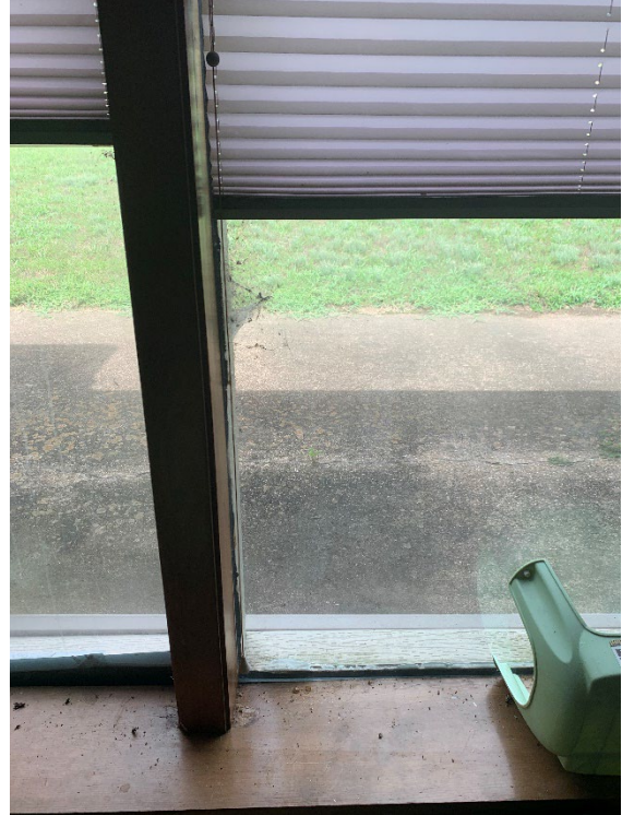
Above: Deteriorated window frame at 1157 Nichols Rd.
