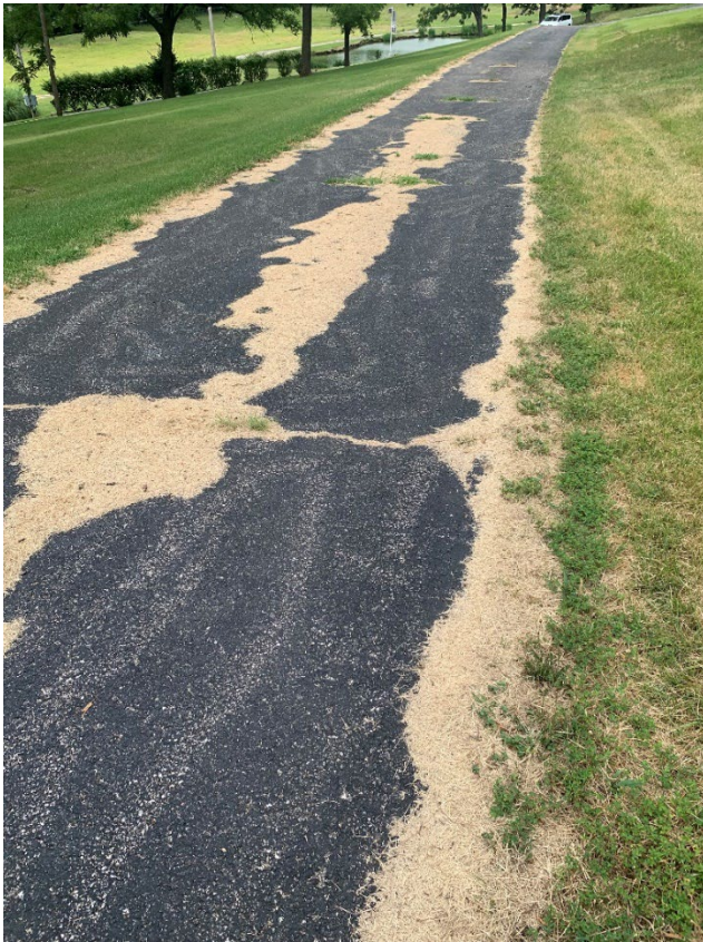
Above: Deteriorated driveway.
