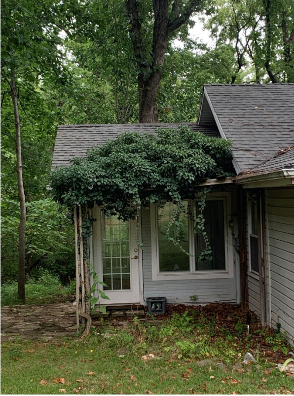
Above: Vegetation overtaking three-season room at 1167 Nichols Rd.
