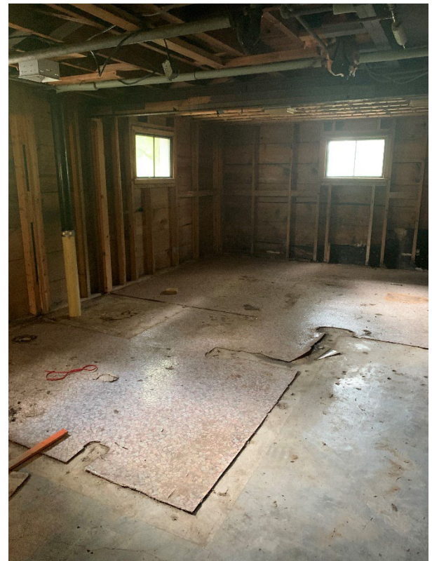
Above: Deteriorated walls at 1167 Nichols Rd.
