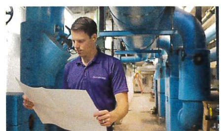
MECHANICAL, ELECTRICAL, PLUMBING
