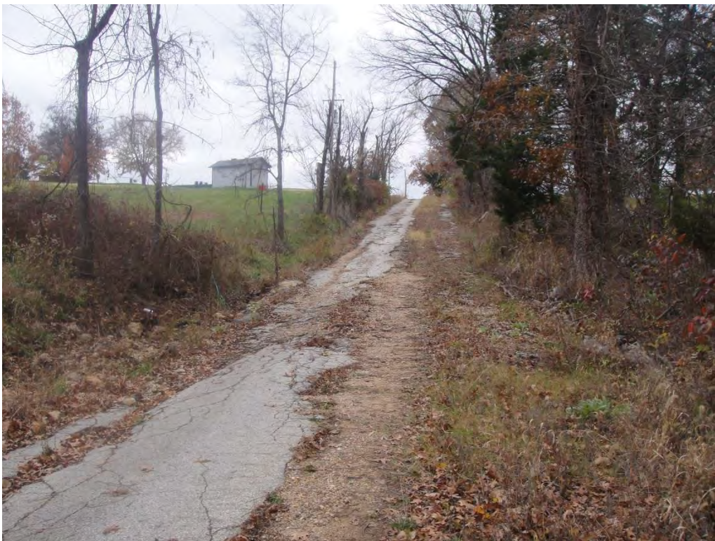
View west along Golf Road. Note significant deterioration, topography differential, limited visibility, lack of curbs/gutters/sidewalks, typical along road.
