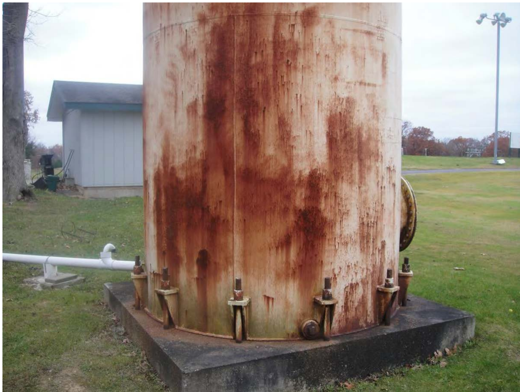
Base of water tower. Note significant surface rust.
